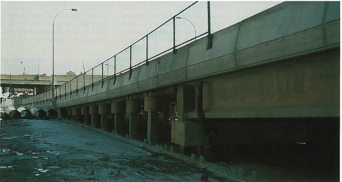
Fig. 7. Pier between the New England bulb-T girder and the slab-on-pile structure. This pier is supported on 12 in. (305 mm) square precast piles.
