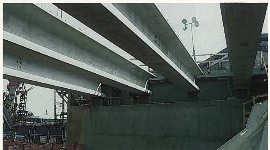
Fig. 5. The 20 ft (6.10 m) high abutment also acts as a transition pier between the New England bulb-T girders and the main structure.
