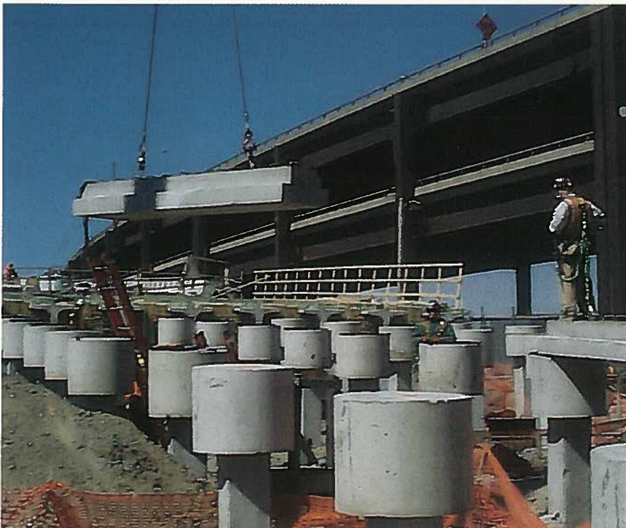
Fig. 3. Placement of T-shaped cross-beams on pile caps for the slab-on-pile transition structures.
