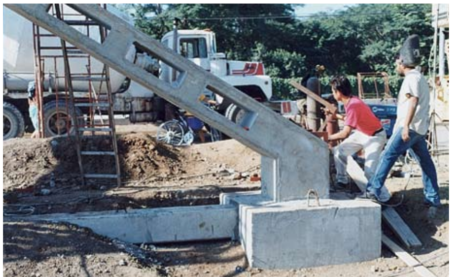
Fig. 14. Upper chord elements of arch, tension footing beam, and pocket foundation connection during erection.
