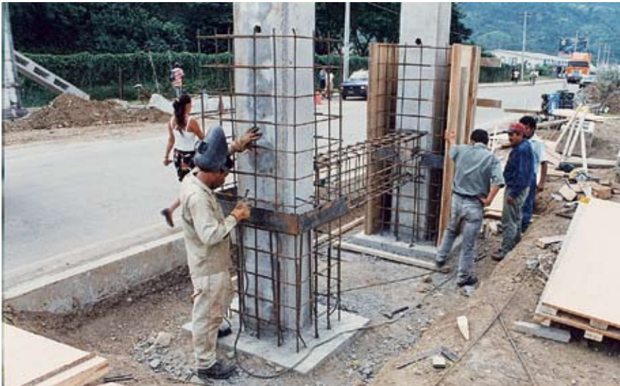
Fig. 10. H-frame columns being fitted with two reinforced concrete collars for strut girder.
