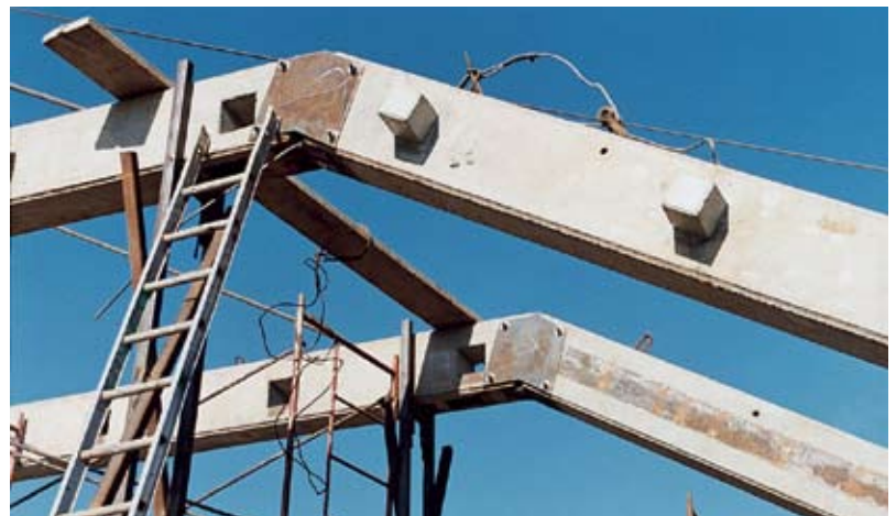
Fig. 19. Connection between main beam and inclined beam using steel plate and bolts.
