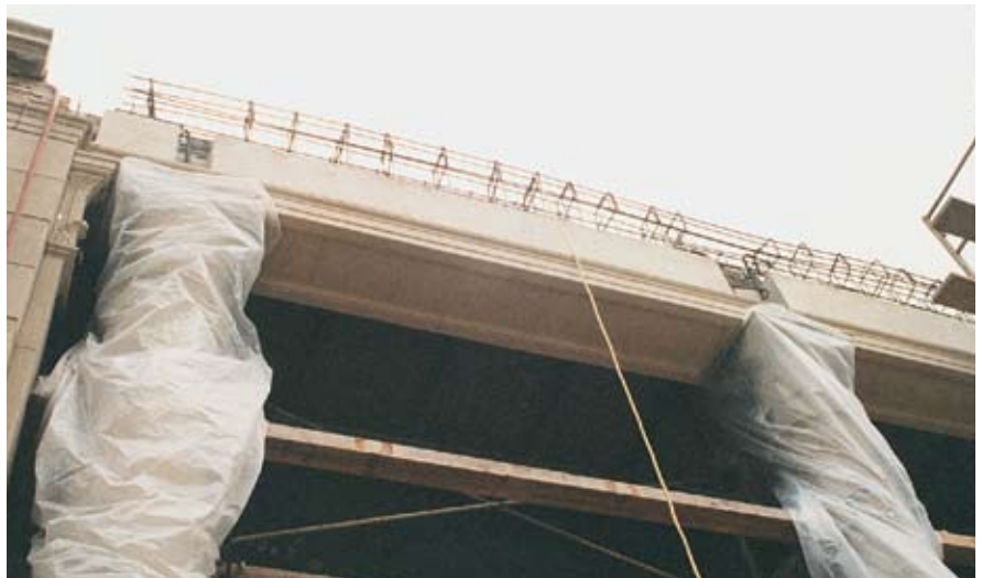
Fig. 5. Erection of the new precast beams. The beam soffits were cast with the same shape, color, and texture as the original damaged limestone soffit.
