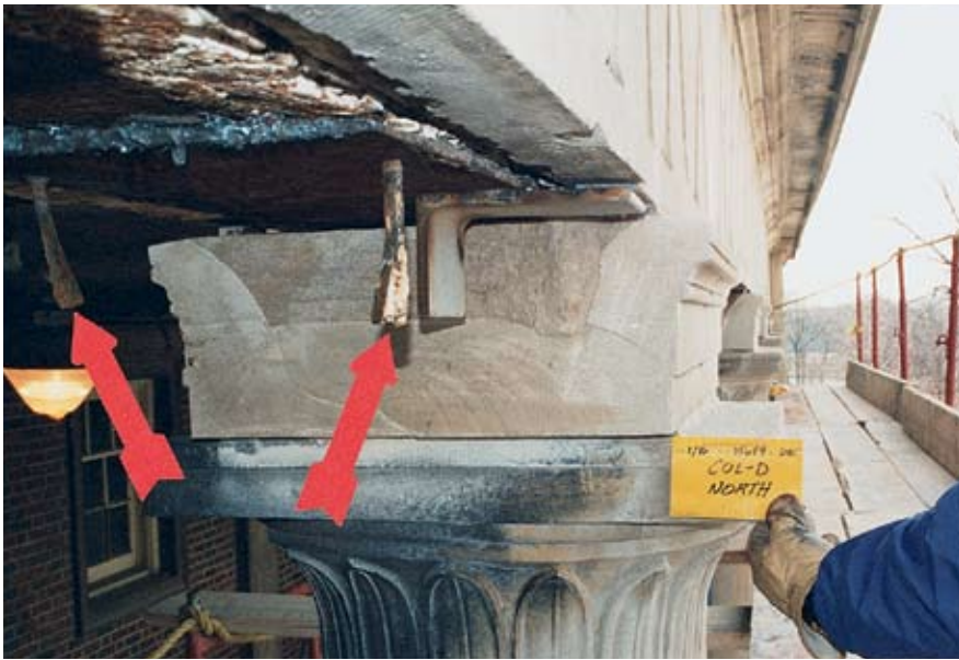
Fig. 3. Damaged limestone soffit that was cut and removed. Arrows indicate metal anchors used to hang the limestone soffit from the supporting steel beams.
