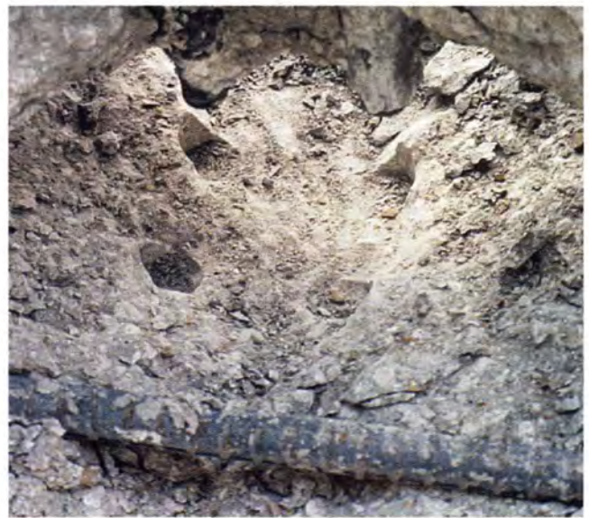
(b) Modified failure plane in concrete.
