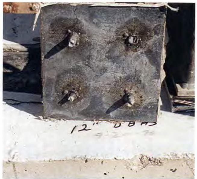
(b) Plate with failed deformed bar anchors.
