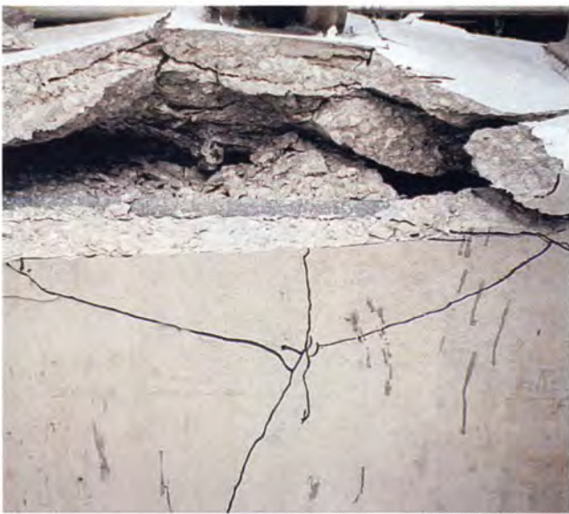
(a) Cracking pattern at concrete failure.
