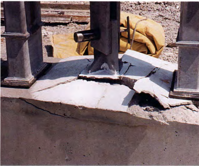
(a) Cracking pattern at concrete failure.
