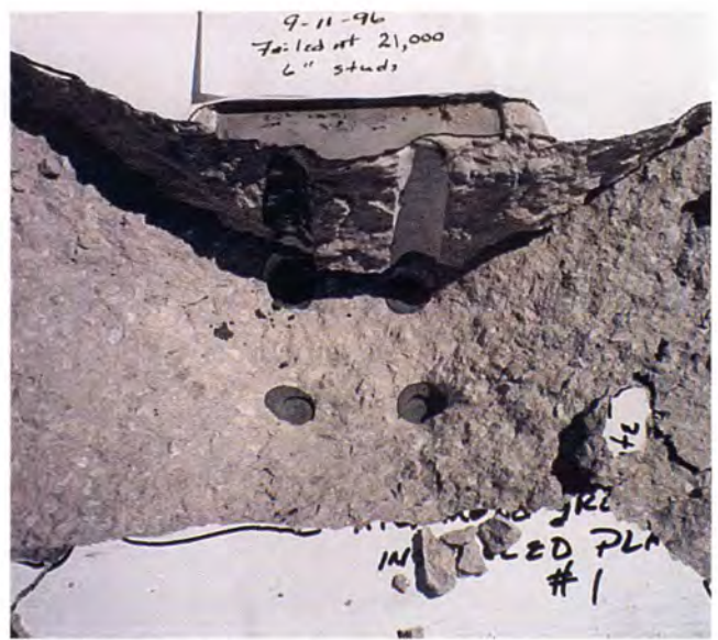
(b) Failure plane in concrete.
