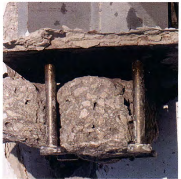
(b) Failure plane in concrete.
