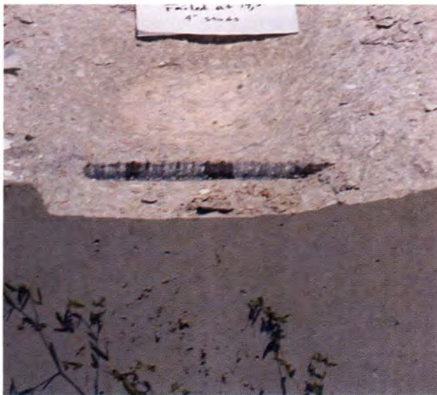
(a) Area after concrete failure cone was removed.
