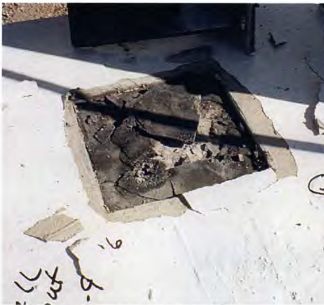
(a) Concrete in the area of the failed plate.
