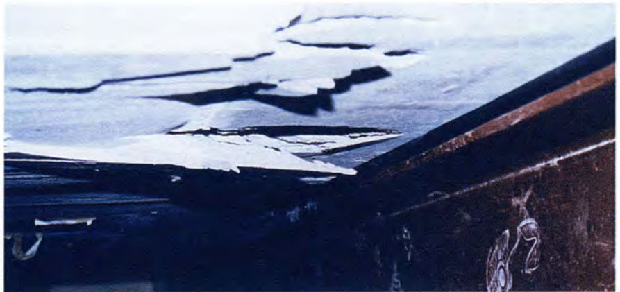
Fig. 17. Shear failure of stems.
