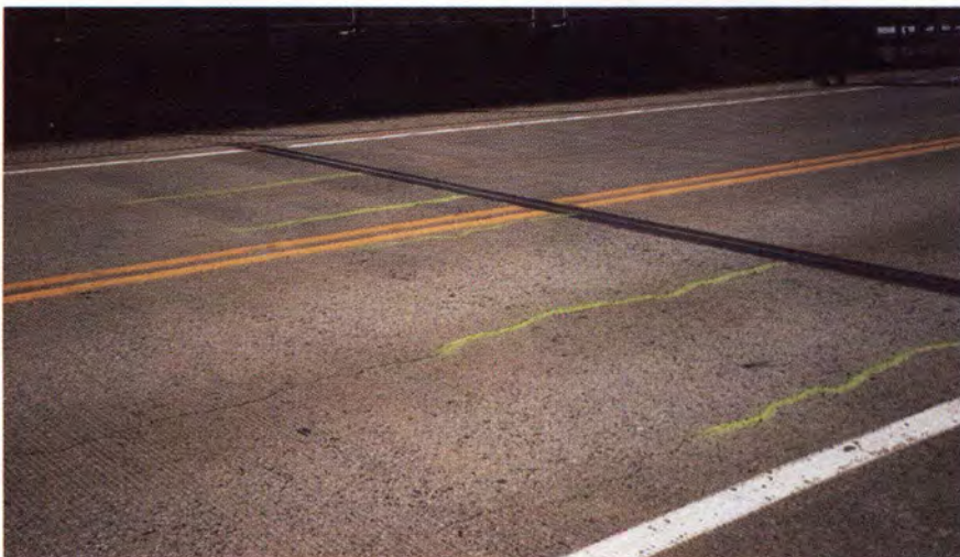
Fig. 4. Typical longitudinal deck cracking over shear keys.
