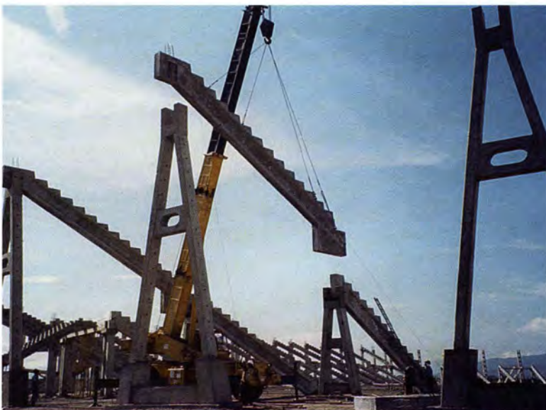
Fig. 12. A-shape column in position as primary beam is being lowered to rest on top of column.
