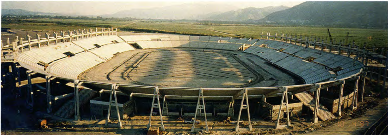
Fig. 1. Aerial view of mid-stage erection of The Olympic Stadium Project in San Pedro Sula, Honduras.
