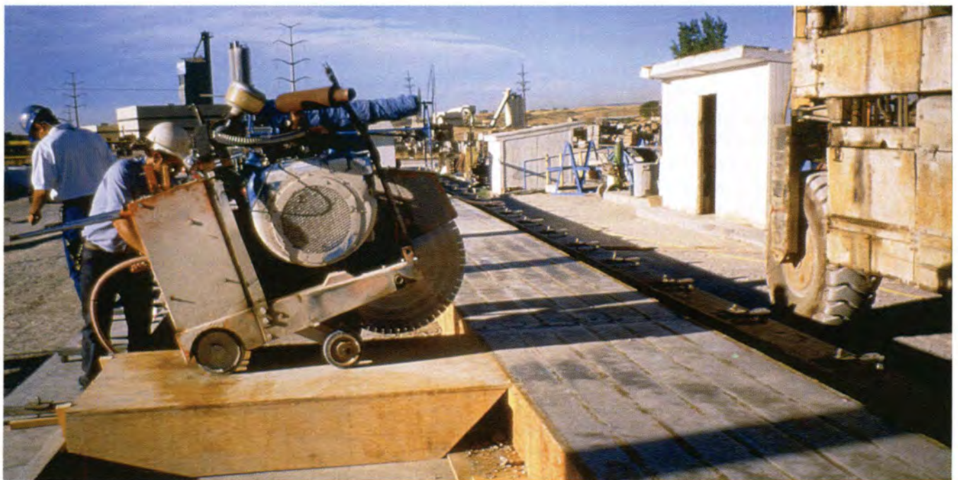
Fig. 14. Release of prestress force by saw-cutting at ends of each 18 ft (5.49 m) beam length (May 18, 1996).
