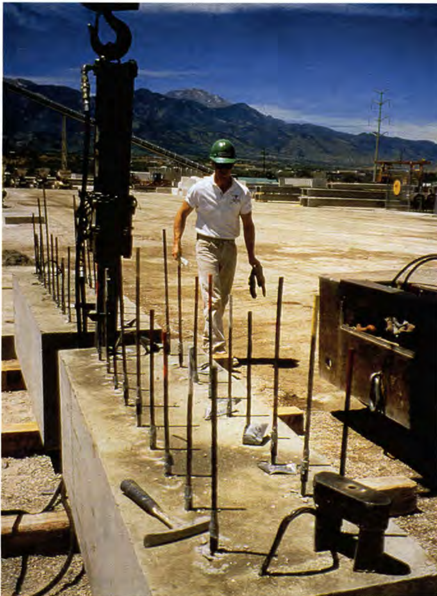
Fig. 17. Strand Groups D and ER pulled out 6 to 8 in. (152 to 203 mm) at 12 kips (53 kN) maximum load. Other groups exceeded 36 kips (160 kN) with less than 2 in. (51 mm) pull-out (May 18, 1996).
