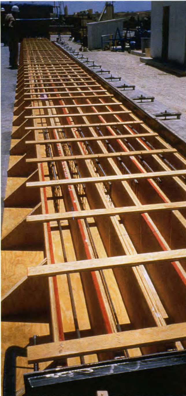
Fig. 11. Wood form, steel end plate, strand and web mesh in place, ready for concrete casting (May 17, 1996).
