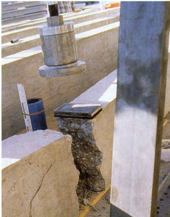
Fig. 27. Strand break, Beam TW-5 (north end). Energy release from 43 kip (191 kN) load in strand caused 6.08 ft (1.85 m) beam end to rebound 6 in. (152 mm) to north (June 8, 1996).
