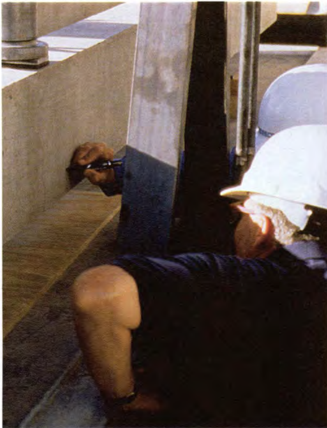
Fig. 25. Detecting and marking first cracks, Beam TW-5, L_e = 6.08 ft (1.85 m) north end (June 8, 1996).
