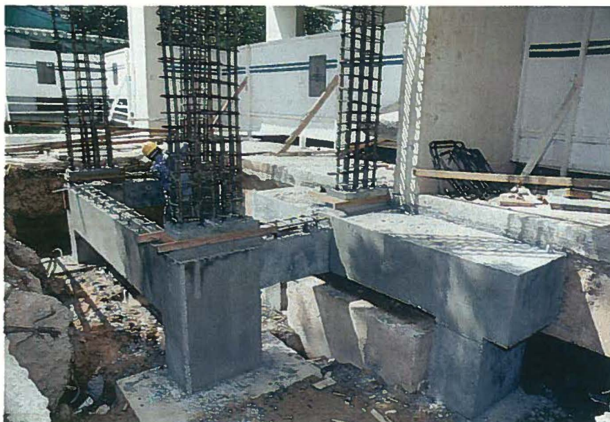
Fig. 3. Foundation for added space showing ground transfer beam layout (Block 413 Clementi Estate).
