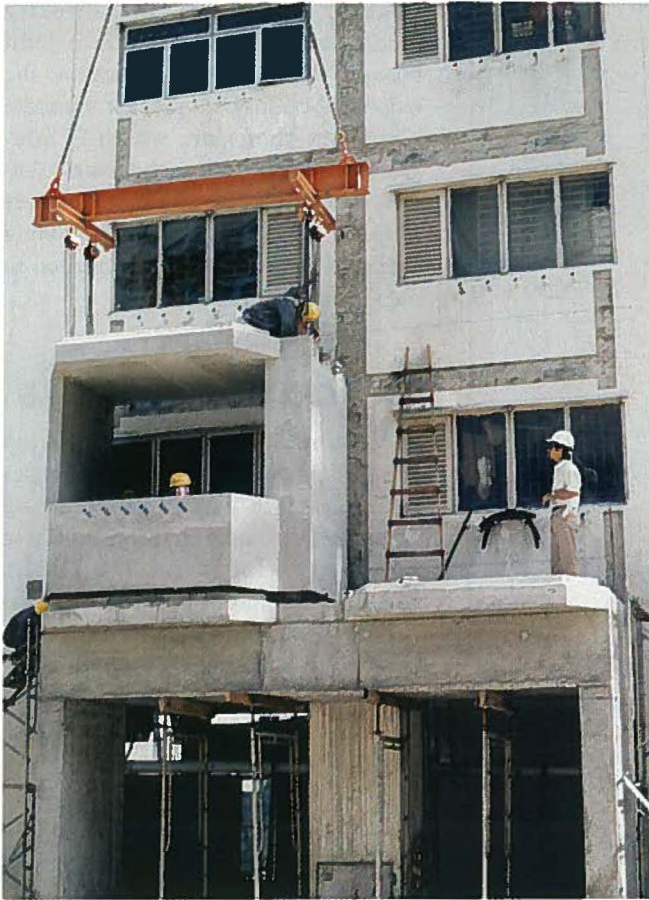
Fig. 14. Precast volumetric (N type) stack supported on transfer beam at second story.
