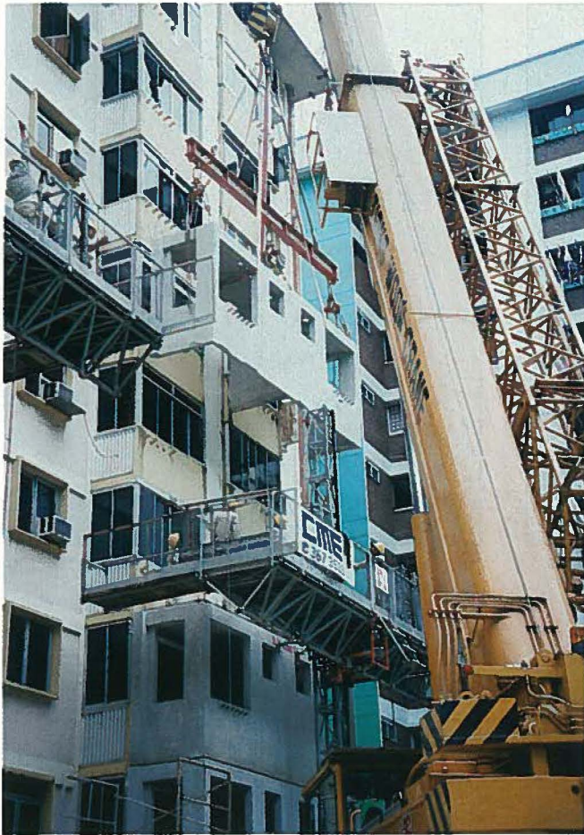
Fig. 12. Precast M Volumetric for two combined units of added space being lifted into position at Block 32 St. Michael's Estate.
