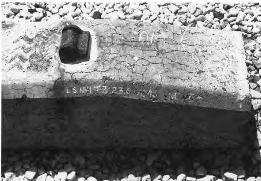
Fig. 1. Precast, prestressed railway tie evidencing DEF induced cracking after several years in service.
