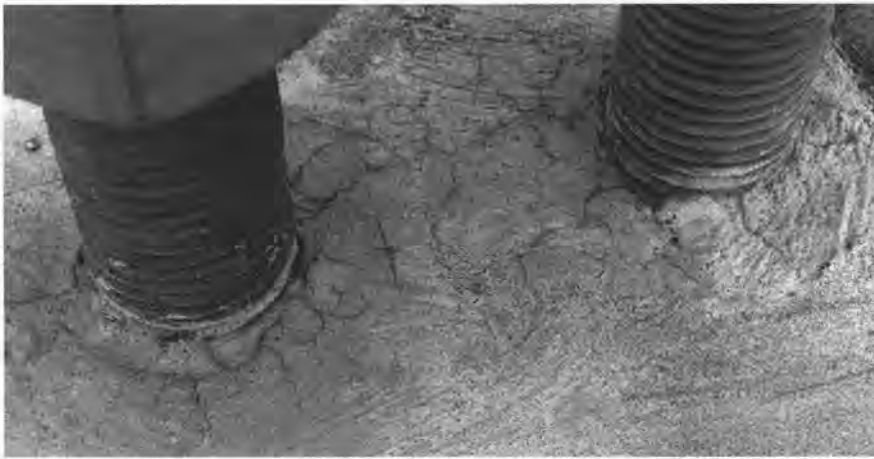
Fig. 3. Cast-in-place concrete piers for electrical transmission lines evidencing DEF cracking about 8 years after installation.
