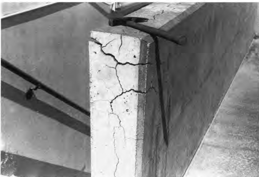
Fig. 2. Precast parking garage wall evidencing DEF induced cracking about 8 years after installation.
