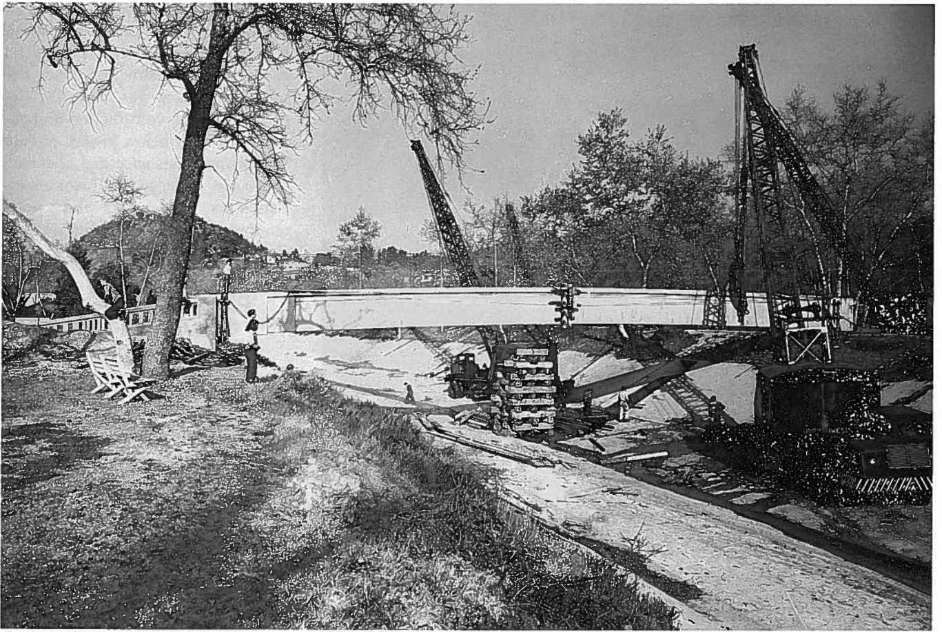
Fig. 1. Construction of the Arroyo Seco Pedestrian Bridge, the first prestressed bridge in California.
