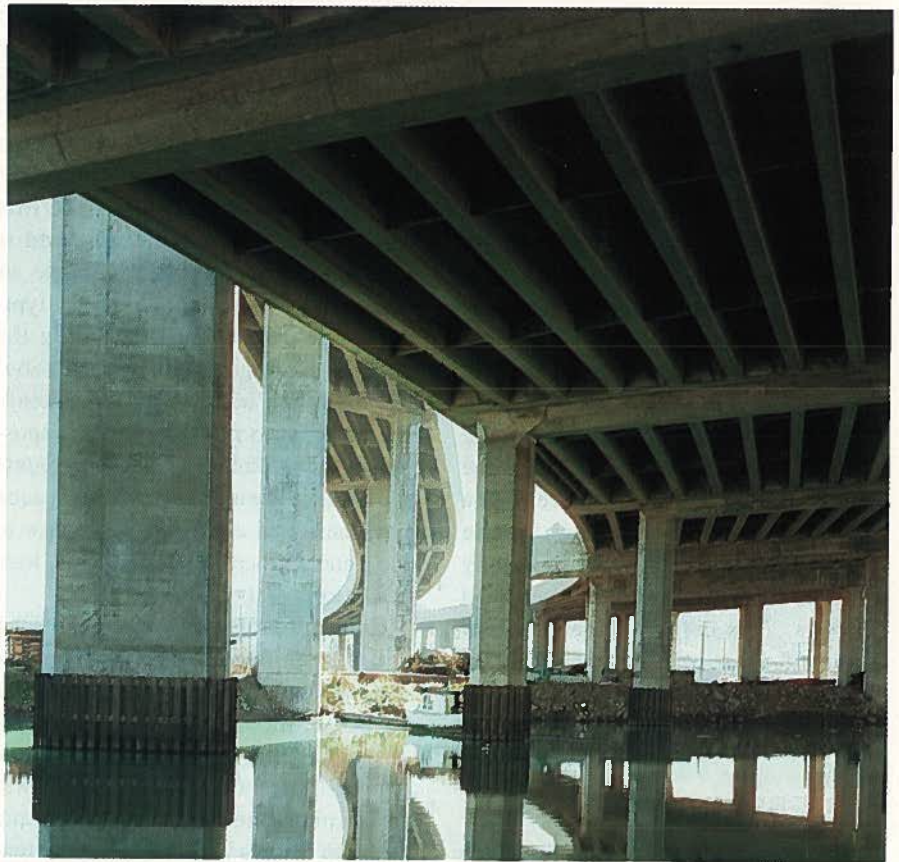
Fig. 4. The Route 280 Viaduct in San Francisco, built in the early 1970s, used large quantities of precast prestressed girders.
