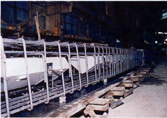
Fig. 14. Reinforcement of box girder. Note: Formation of void using expanded polystyrene, location of diaphragm and positioning of shear reinforcement on a skew angle.
