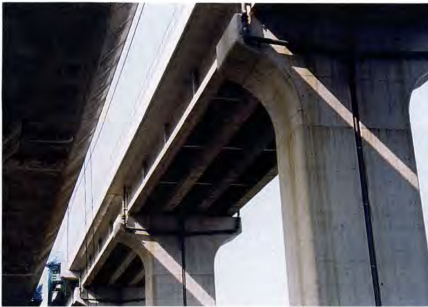
Fig. 19. Completed bridge using post-tensioned T-girders. Note: Cast-in-place diaphragms and narrow girder spacing.
