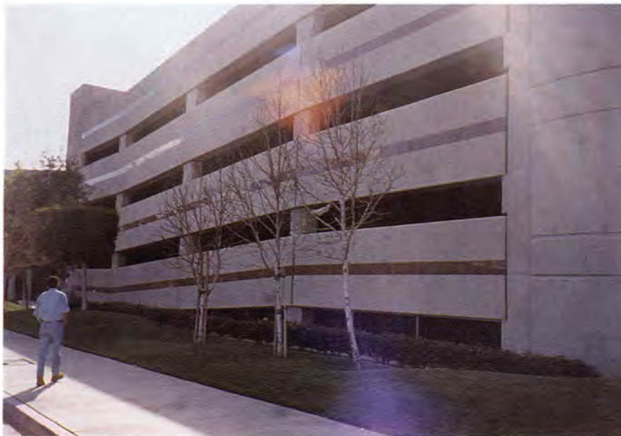
Fig. 11. Coldwell Banker garage, Granada Hills, with mildly damaged column haunches and cracked filler walls about 3 miles (5 km) east of epicenter (Garage 21).
