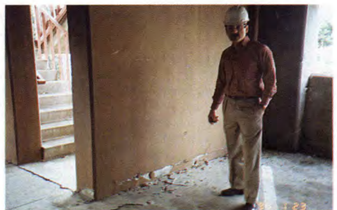
Fig. 16. Glendale Fashion Center. Note failure of shear wall construction joint and of connection of diaphragm to shear wall in northwest corner of second supported level (Garage 6).
