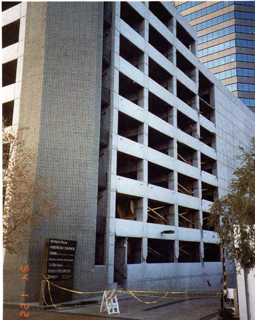
Fig. 23. Garage at southeast corner of Sepulveda and Ventura Boulevards. Damage is due to inadequate separation of precast cladding from columns (Garage 11).
