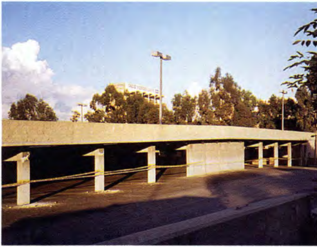
Fig. 24. Sherman Oaks Galleria-East Garage. South face shows form of garage and cosmetic damage at exterior beam-to-column connections (Garage 9).
