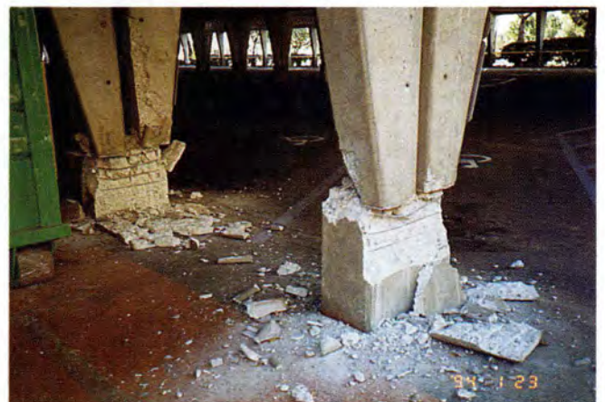
Fig. 21. Glendale Galleria, Columbus Avenue Parking. Spalling of cast-in-place pedestals caused settlement of tables (Garage 8).
