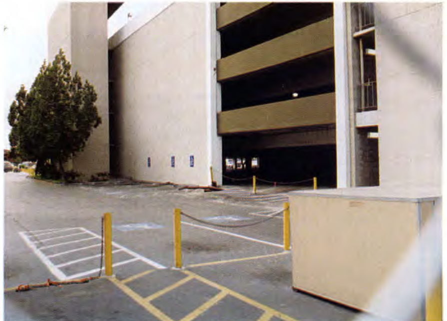
Fig. 29b. Kaiser Permanente, West Los Angeles-West Garage. Note uplift of spread footing of east shear wall and separation of stairwell tower from shear wall (Garage 14).
