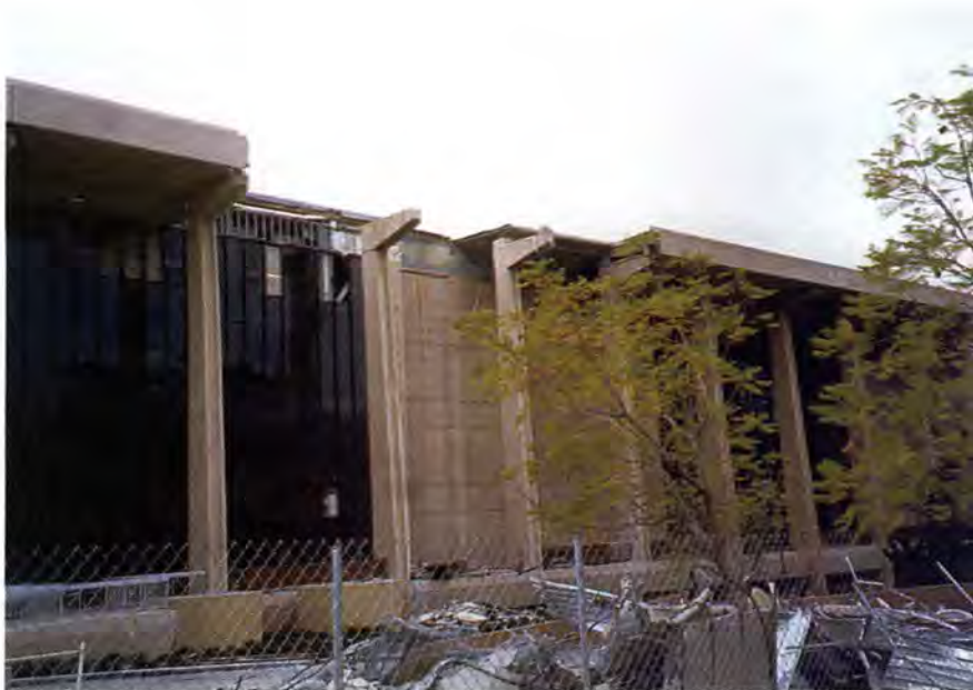
Fig. 33. Roof failure at Oviatt Library, CSU-Northridge.
