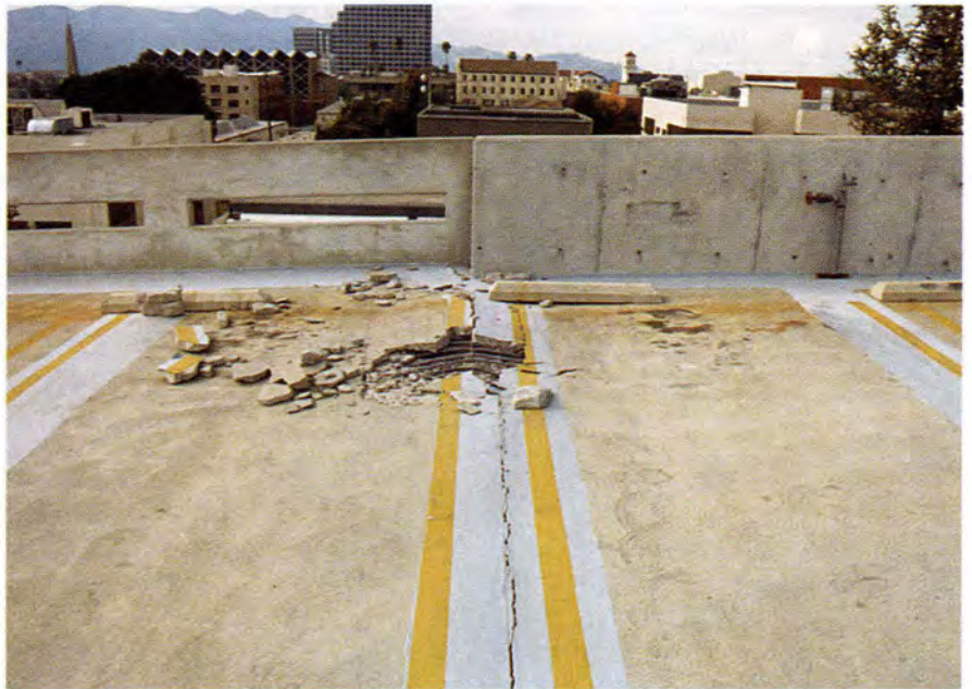
Fig. 19. Glendale Civic Center. Fracture line extending across diaphragm to area of crushing and bar buckling on west side (Garage 7).
