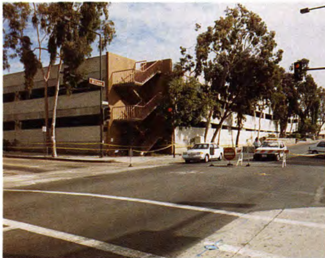
Fig. 13. Glendale Fashion Center (southwest corner). Lower story columns on right have shortened markedly compared to upper story columns (Garage 6).
