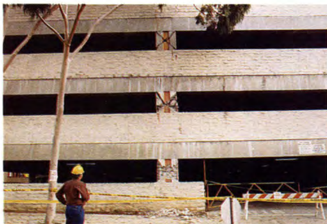
Fig. 14. Glendale Fashion Center. Note "short column" cracking on west face (Garage 6).
