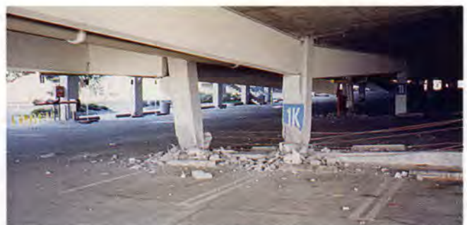
Fig. 9. Gravity load interior columns, southwest corner, CSU-Northridge garage showing crushing of column bases and incipient failure of floor due to loss of support for transfer beams (Garage 5).
