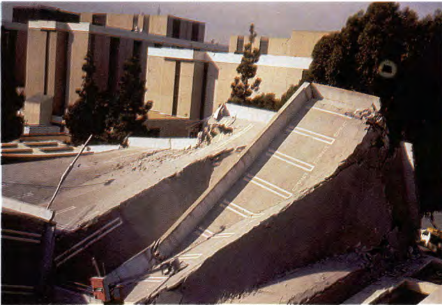
Fig. 28. Kaiser Permanente, West Los Angeles-East Garage. Shows a view of the collapsed structure looking west in a direction parallel to the frames (Garage 13). (Courtesy: Portland Cement Association).
