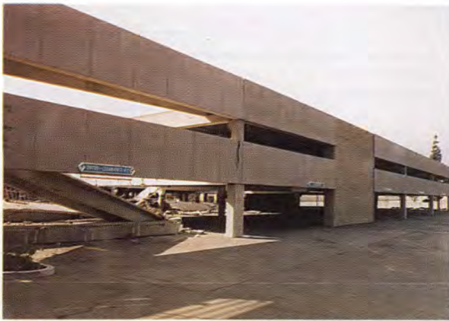
Fig. 4. North face of northwest garage at Northridge Fashion Center with partially collapsed area at left (Garage 2).
