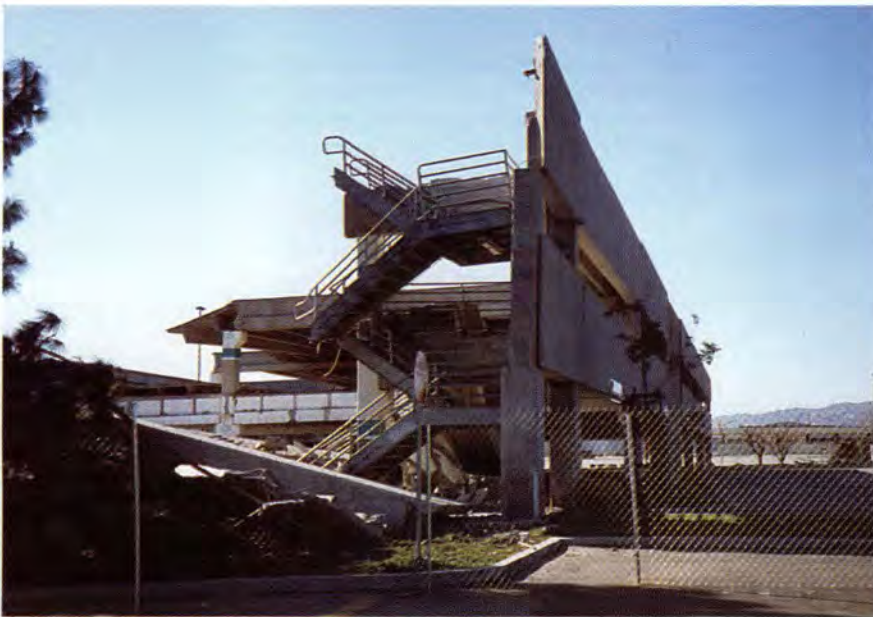
Fig. 6. Collapsed northeast corner of northwest garage of Northridge Fashion Center showing precast concrete column, spandrel panel and floor details (Garage 2).
