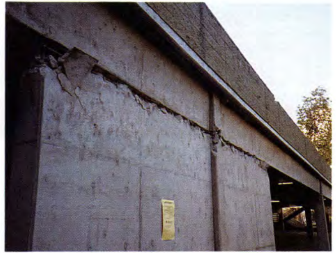
Fig. 25. Sherman Oaks Galleria-East Garage. East face shows failure at shear wall to frame connection and yellow tagging of structure (Garage 9).
