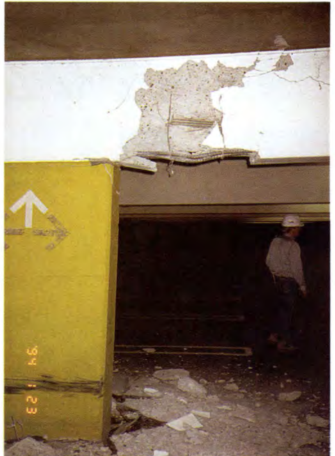
Fig. 27. Sherman Oaks Galleria-South Garage. Note damage to beam at connection to interior shear wall on spread footing (Garage 10).
