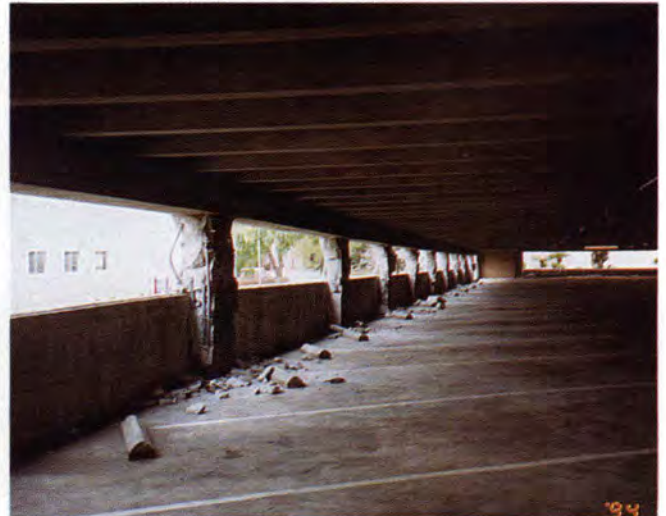
Fig. 15. Glendale Fashion Center. Interior view along north face shows double tee floor and column cracking/bar buckling along north face (Garage 6).
