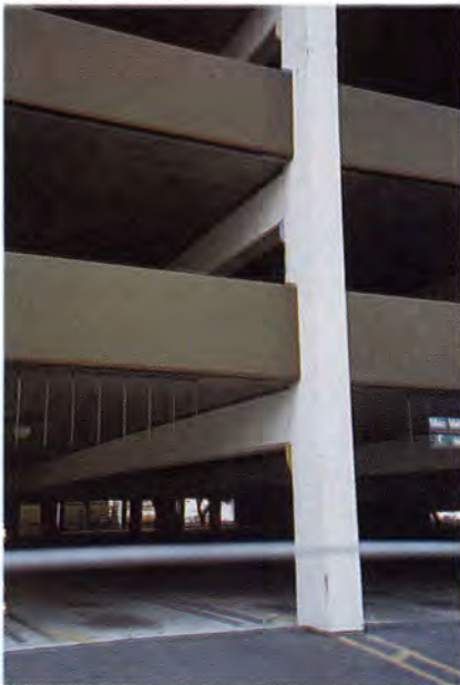
Fig. 29a. Kaiser Permanente, West Los Angeles-West Garage. Shows damage to exterior columns on north face (Garage 14).
