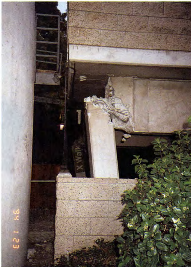
Fig. 26. Sherman Oaks Galleria-South Garage. Note fracture of exterior column in northwest corner of gravity load frame (Garage 10).
