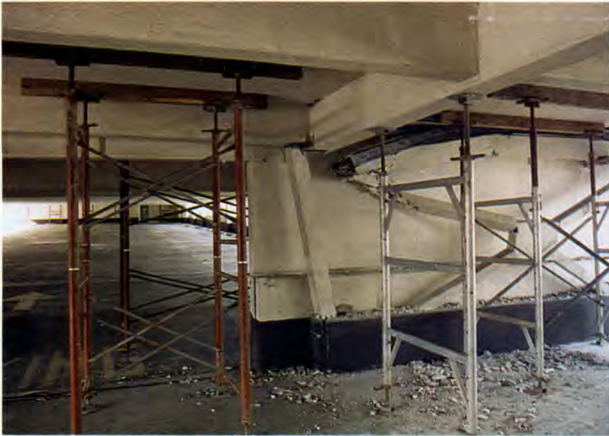
Fig. 30. St. John's Hospital, Santa Monica. Fracture and buckling of braced steel frame of center garage (Garage 18).
