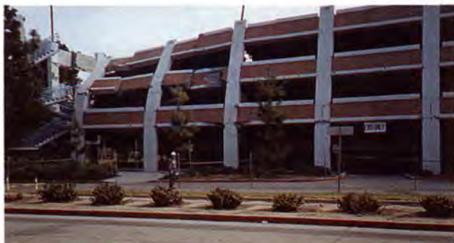
Fig. 8. Northwest corner of CSU-Northridge garage showing gravity load column trees separating from each other as diaphragm fails (Garage 5).
