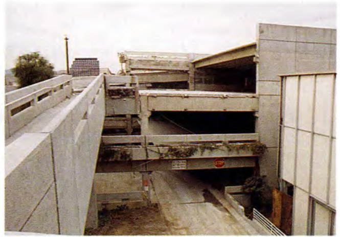
Fig. 18. Glendale Civic Center. Collapsed roof and floor areas on east side (Garage 7).
