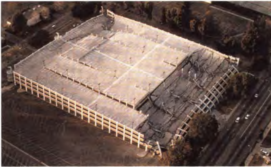
Fig. 7. Partially collapsed garage at CSU-Northridge looking north (Garage 5). (Courtesy: Engineering News-Record ).
