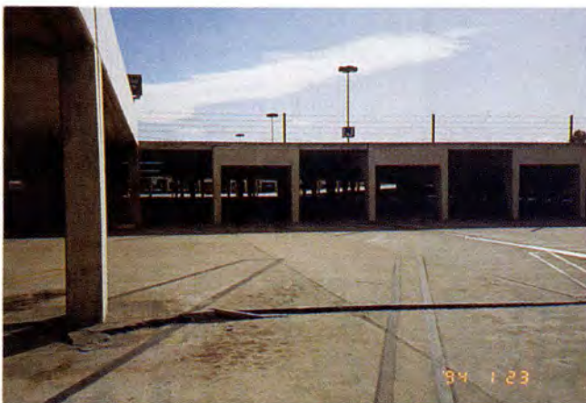
Fig. 20. Glendale Galleria, Columbus Avenue Parking. Roof level shows precast concrete "Conrad tables" and settlement at joint line (Garage 8).
