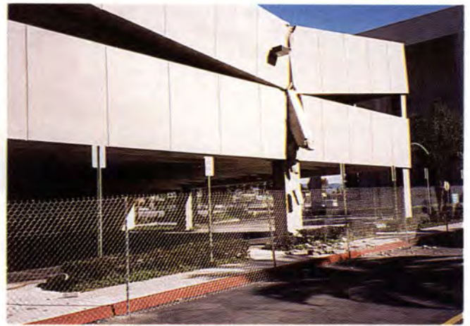
Fig. 5. Collapse of second-story portion of precast concrete column on south face of northwest garage at Northridge Fashion Mall (Garage 2).
