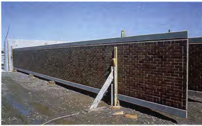
Fig. 17. A vertical easel was an effective restraint for 65 ft (19.8 m) long prestressed concrete panels during stockpiling.
