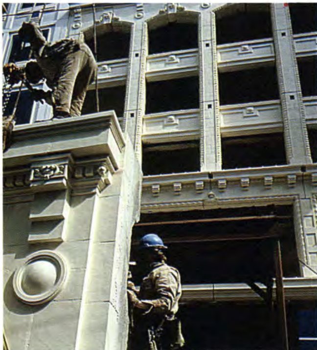
Fig. 10. Built in 1906, the six-story 88 Kearney St. is considered one of San Francisco's architectural landmarks. For that reason, it was decided that the building's terra cotta facade would be preserved on an otherwise all-new structure of slightly taller height. The terra cotta was taken off the building, piece by piece, and the pieces were identified for subsequent reassembly on new precast concrete panels. Architect: Skidmore, Owings and Merrill, San Francisco, California.
