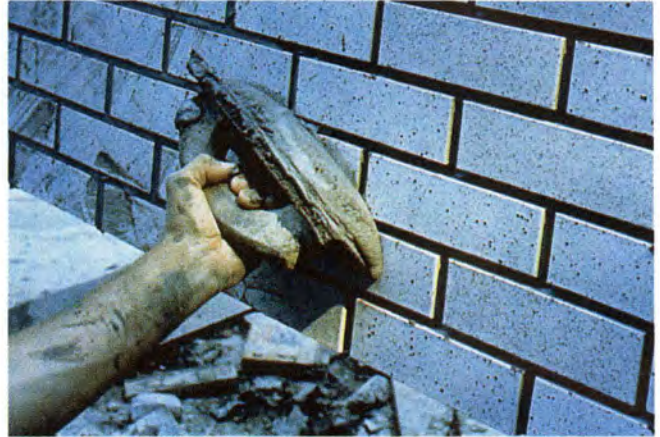
Fig. 20d. Grout is placed into the joints using a baker's bag or large caulking gun. Excess grout is struck from the brick surface using a rubber-faced float. The float is worked at 45 degrees to the surface.
