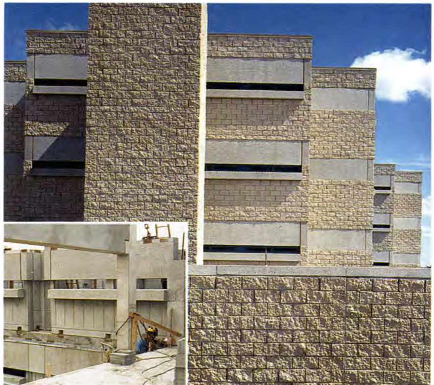
Fig. 25. Panels for the Oakland County Jail Addition in Pontiac, Michigan, were delivered to the site complete with slots for dovetail anchors to support split face block. Architect: NSA-HDR — A Joint Venture, Southfield, Michigan.
