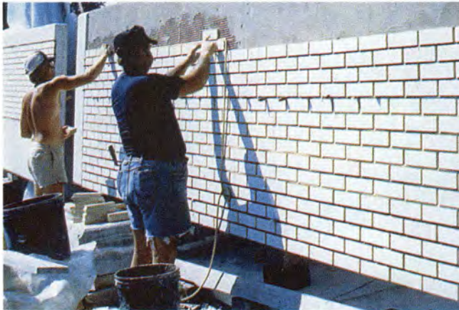
Fig. 20b. A second coat of mortar is applied to the panel surface using a notched trowel. The glazed brick is then applied to the panel surface.
