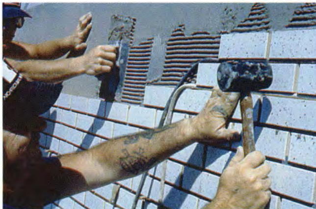
Fig. 20c. The bricks are tapped into the mortar using a rubber mallet. Level and alignment are also checked at this point.
