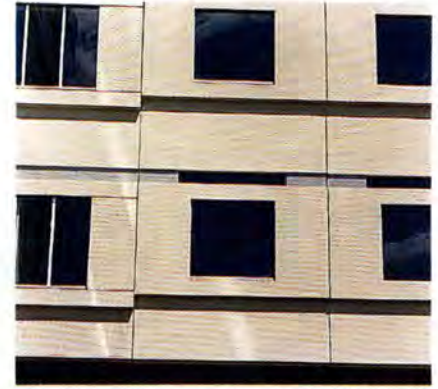
Fig. 21b. The paper-faced 2 in. (50 mm) square tiles on a 1 ft (0.3 m) square sheet were applied in the plant using latex-portland cement mortar and easily adapted to the complex wall profiles.
