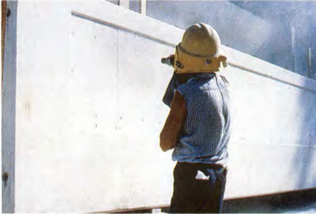
Fig. 20a. The surface of the panel is lightly sandblasted prior to parging with a skim coat of latex-portland cement mortar.
