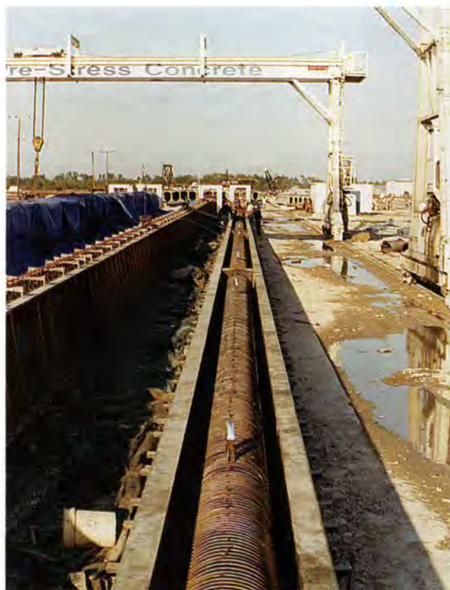
Fig. 2.12. Congestion with heavy spiral reinforcement.
