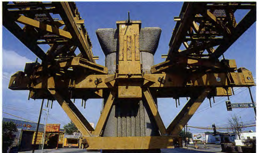
Fig. 20. Erection trusses are supported on steel brackets suspended from and clamped to the piers.
