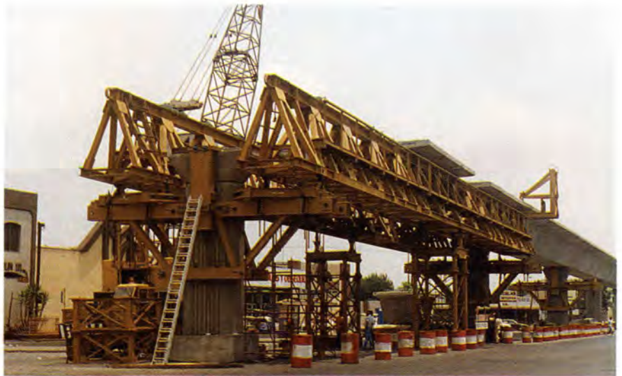
Fig. 19. Full-span erection trusses support the segments for a span until all are placed, post-tensioned and set on the pier bearings.
