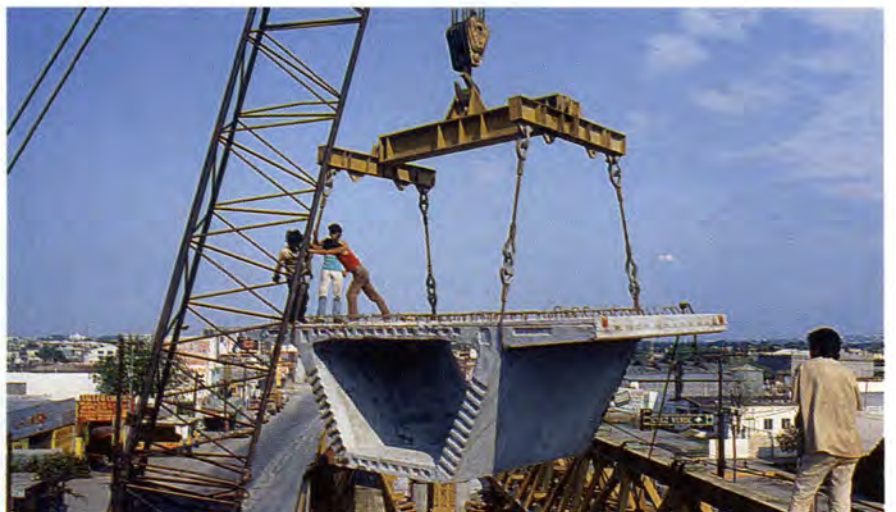
Fig. 21. Segments are lifted from street level by crawler cranes and set on erection trusses.
