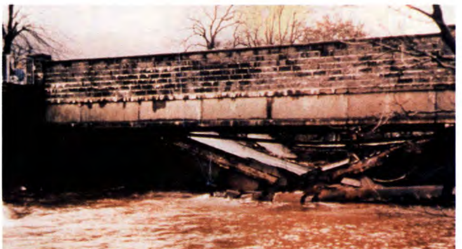
Fig. 10. Collapsed Ynys-y-Gwas Bridge (from Ref. 1).
