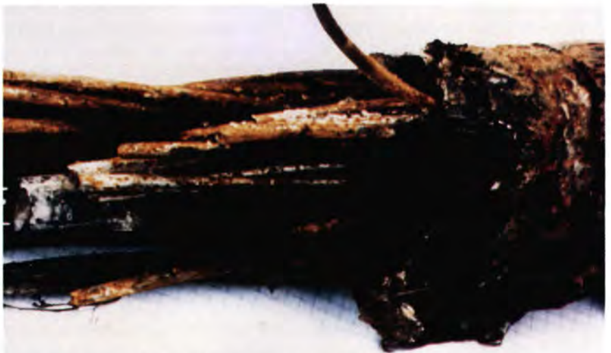
Fig. 15. Corrosion failure of a ground anchorage (Courtesy of Peter Matt).
