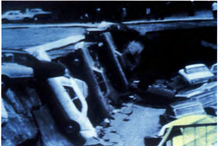
Fig. 9. Parking garage failure resulting from corroded tendons (Courtesy of Florida Wire and Cable Company).
