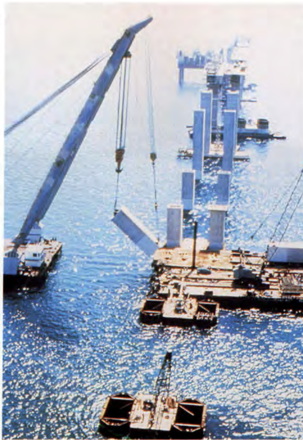
Fig. 5. Erecting precast concrete segments for the King Fahd Bridges between Saudi Arabia and Bahrain.
