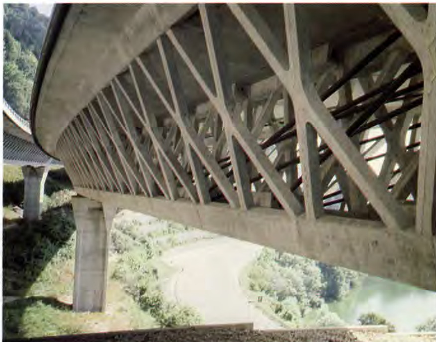
Fig. 8. Elegant and efficient truss of high strength precast concrete segments, joined by post-tensioning.
