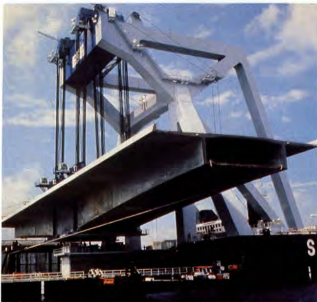
Fig. 6. 6000 ton prestressed girder, 104 m (308 ft) span for Great Belt Western Bridge, Denmark.
