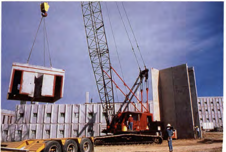
Precast module (weighing 27 tons) being lifted into place. Each 176-cell four-story housing building was erected in less than 30 working days.
