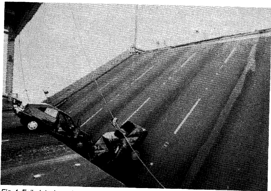
Fig. 4. Failed deck section of Bay Bridge (from Engineering News-Record report).
