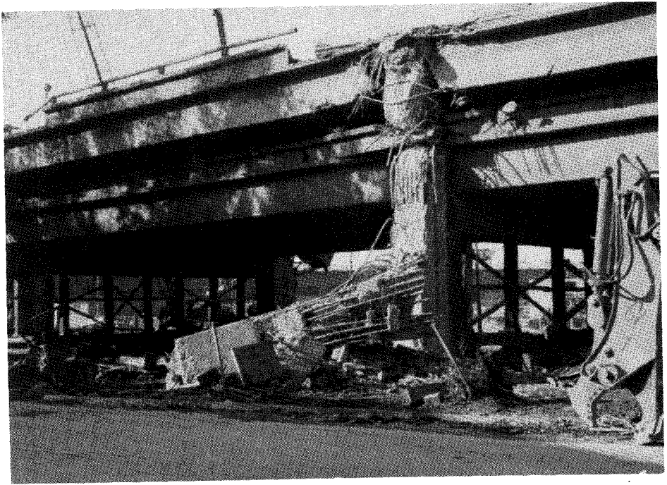
Fig. 3. Collapsed portion of I-880.
