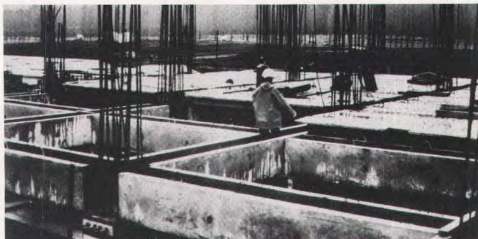
Fig. 3. Precast concrete U-beams used as permanent formwork for cast-in-place reinforced concrete frames (Karioi Pulp Mill Building, New Zealand).
