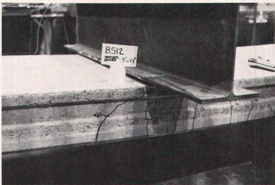
Fig. 2. Inclined shear cracking of hollow-core specimen.
