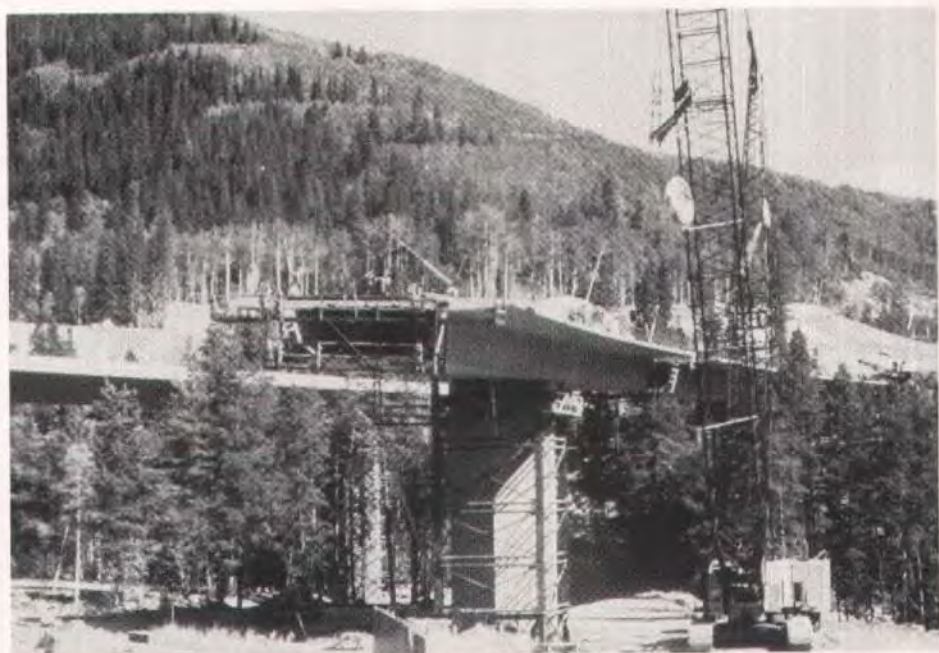
Fig. 1b. Precast segmental box girder bridge being erected in balanced cantilever fashion using a crawler crane.
