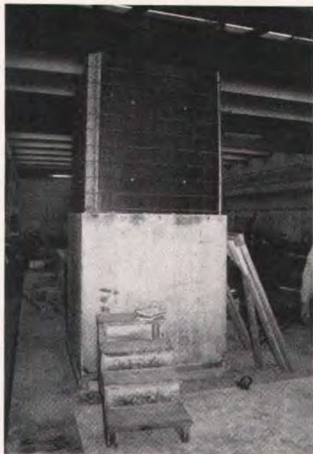
Fig. 25. Forming of match-cast segment which was post-tensioned to adjoining segments before being moved to the testing lab.
