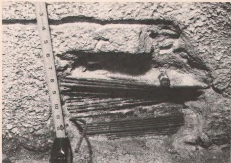
Fig. 4. Corroded wires bundled around a pipe. Shotcrete protection did not penetrate bundle and was not bonded to tank wall.
