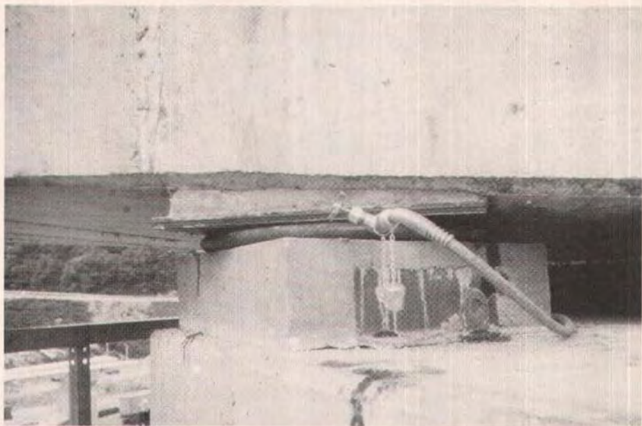
Fig. 23. Flat jacks were used to set the structure to elevation and to grade.
