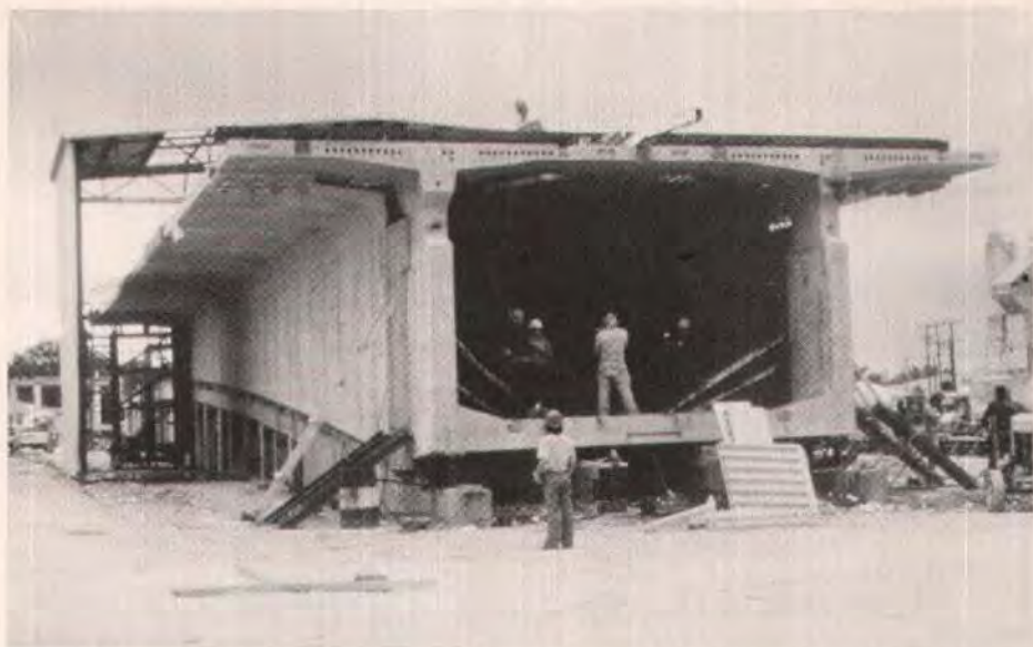
Fig. 12. A previously cast segment was brought back and positioned as in a short-line bed in order to cast the pier segment.
