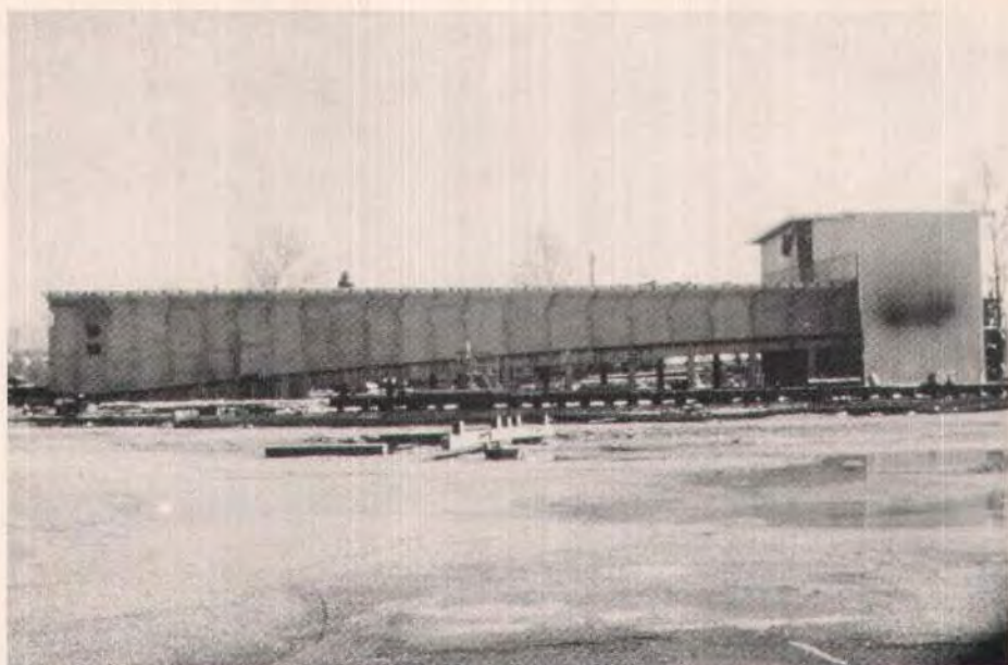
Fig. 14. A work shed was placed over the bed so that production continued in bad weather. Average production was over four segments per week until all 244 were made.
