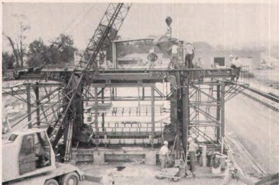
Fig. 10. First segments were produced by placing concrete with a bucket. Later the concrete was pumped into place.
