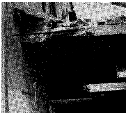
Fig. 17. "Friction Connection" of a lateral beam to a tiltup bearing wall. Note that the angle beneath slab was added subsequent to original construction.
