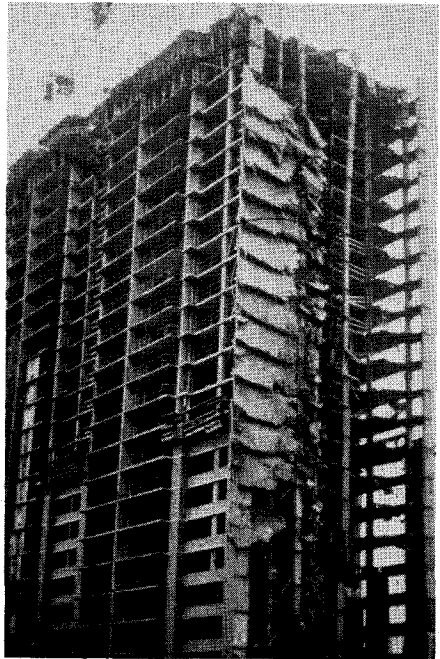
Fig. 6a. Cast-in-place concrete apartment collapse (Bailey's Crossroads, Virginia). Vertical propagation occurred from a shoring error on the upper stories of building.
