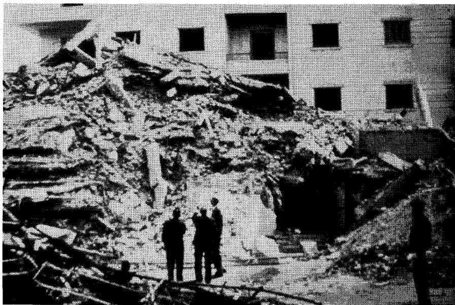
Fig. 12. Egyptian apartment building after loss of a foundation. Note that building is identical to one in background.
