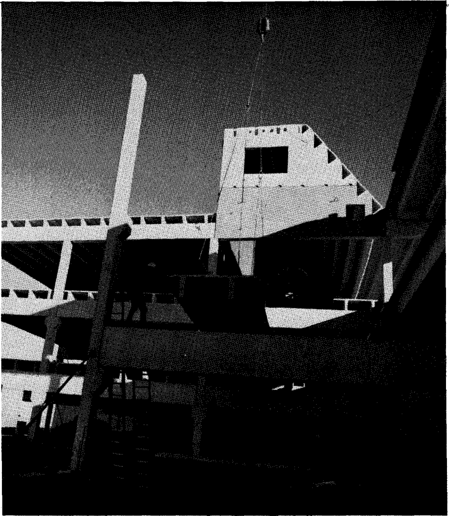
Overall shot of structure during erection; double tee is being lowered into position.
