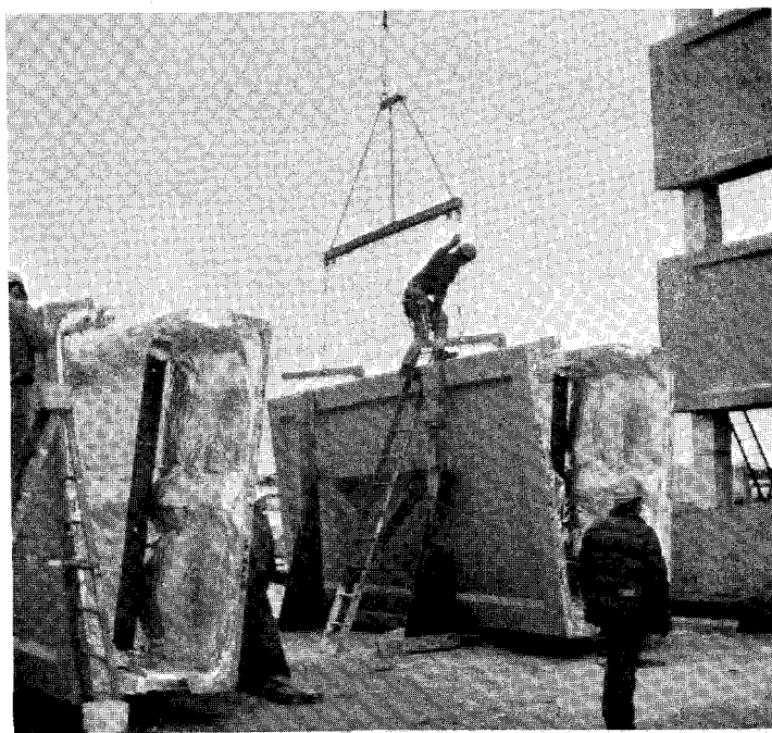
Fig. 25. Panels at RCA job site being readied for placement on building. Panels were insulated at producer's plant for a "U" factor of 0.05. Typical panels are 20 ft x 9 ft 6 in. x 2 ft deep and weigh 2800 lbs. (Courtesy: Olympian Stone Company.)
