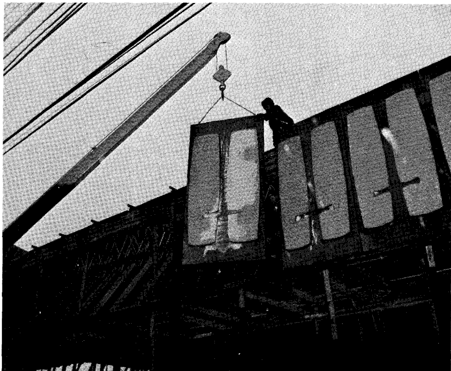
Fig. 22. Fascia panels are lifted into place on to wood framing at U.S. Post Office construction site. (Courtesy: Olympian Stone Company.)
