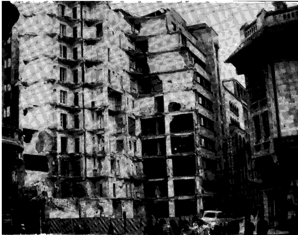
Many pre World War II buildings suffered serious collapse. At the time of construction, seismic design criteria were not established.
