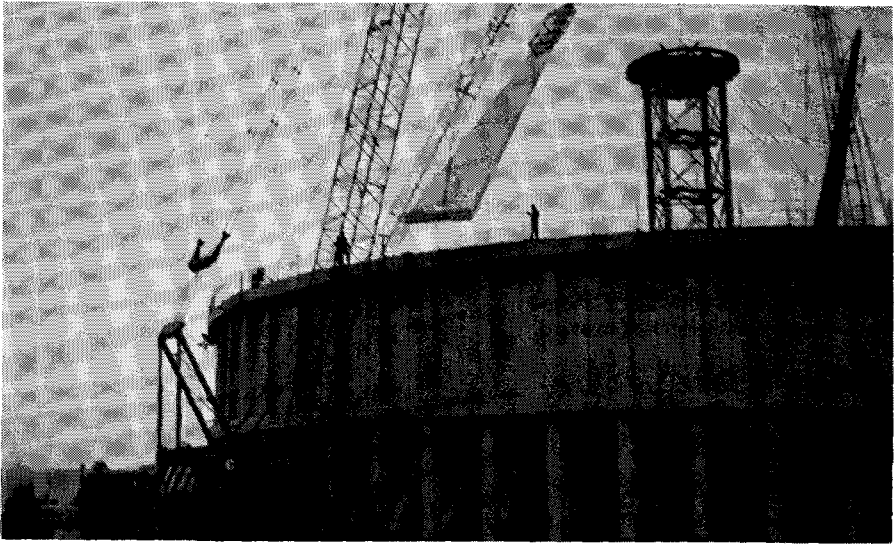
Fig. 17. First two roof units being lifted into place. Note that the segments were erected in pairs to keep the structural loads balanced.
