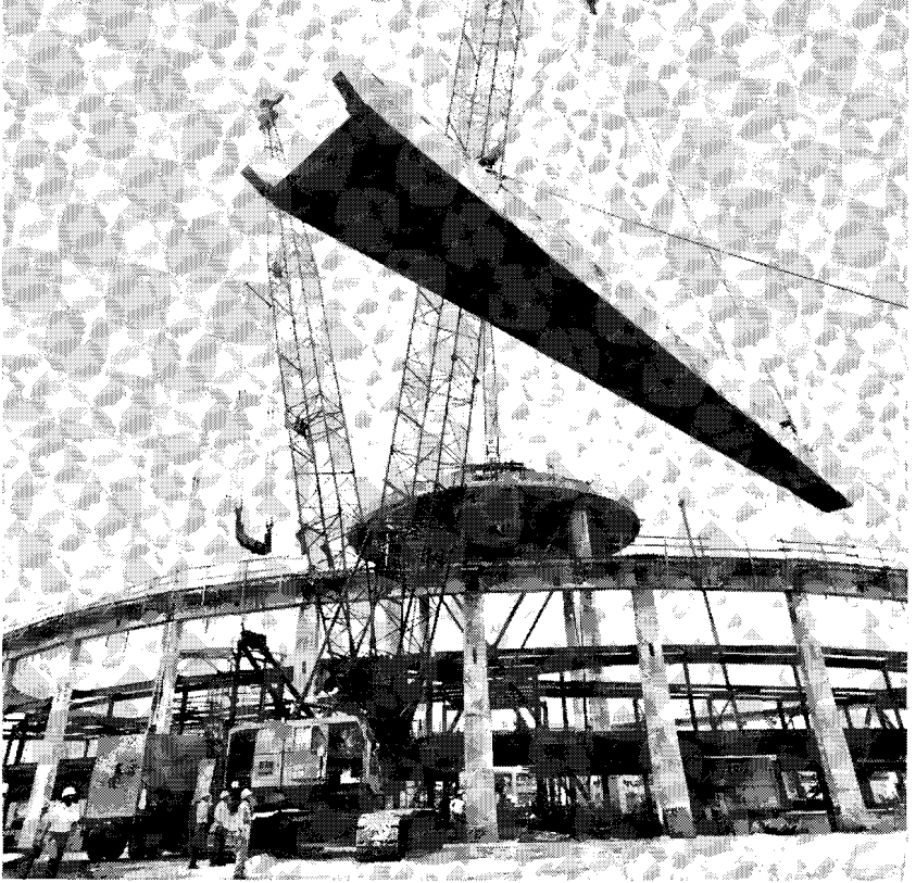
Fig. 7. Placement of first roof channel. The X-bracing of center columns now replaces the guying wires. The crane outside is the American Sky Horse. A special derrick on the center slab will pick up the top end when the channel is inside. The channels weighed about 75 tons apiece.
