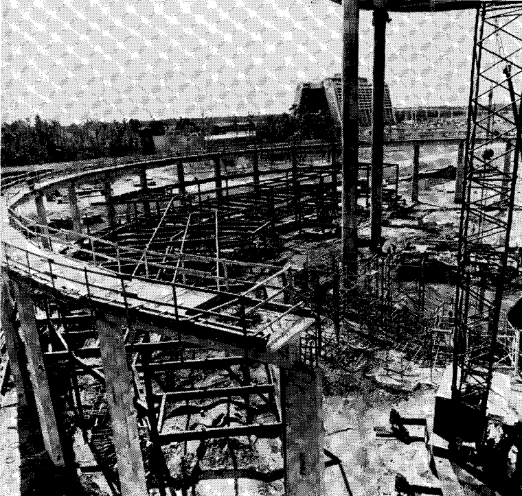
Fig. 6. Ring beam installation. Note that the ride structure is being erected simultaneously.
