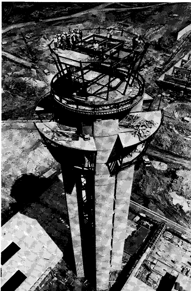
Fig. 6. Modules are stacked to 180 ft and topped by 16-ft high, 11-sided steel cabs and equipment level. Structural steel platforms were set at 15-ft intervals to connect the four service cores.
