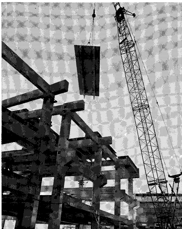
Fig. 9. 18-in. precast double-tee unit being hoisted into position longitudinally and transversely in both floor and roof system.
