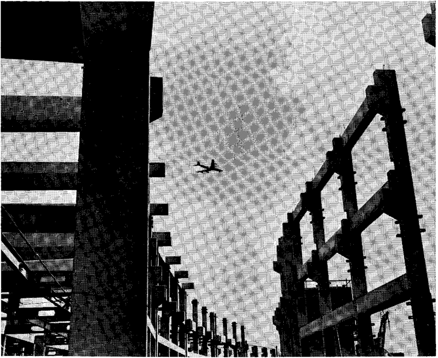
Fig. 8. Terminal building (2W). Primary structural system used precast beam and column frames in both longitudinal and traverse directions. For architectural considerations haunches were eliminated for longitudinal beams. Shears and moments were transferred from beams to columns using shear keys. Continuity in the longitudinal direction was provided using Cona multistrand tendons pulled into place after precast erection.
