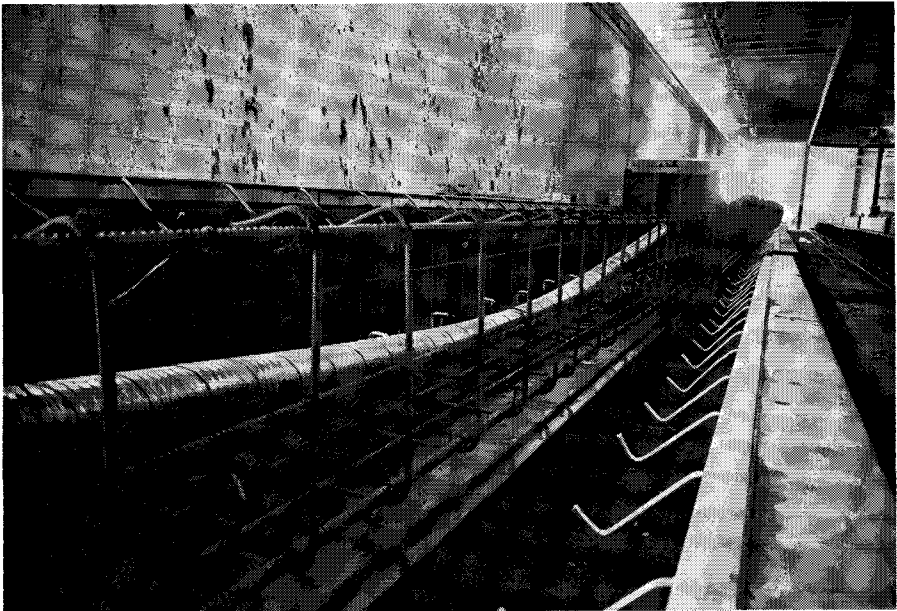
Fig. 11. Precast longitudinal frame beams were pretensioned for their own dead load and handling. Note that the 3/4 in. diameter draped tendon duct was placed in the beam at time of casting. Multistrand tendon was pulled into position in field to create one and three-span rigid frames.
