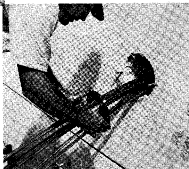
Fig. 21. Spray plates were placed on the tendons to separate the 9-strand tendon into three groups of 3 strands.
