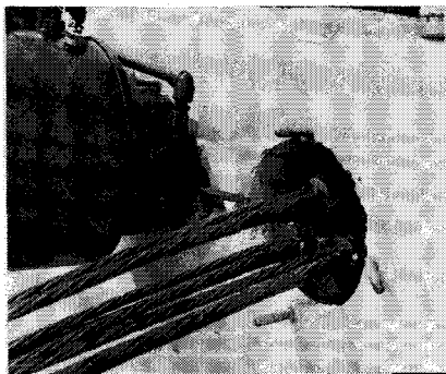
Fig. 22. Closeup of a fully stressed and anchored 9-strand tendon. Jack in place will stress and anchor adjacent tendon. Excess of strands are cut off with an abrasive saw.
