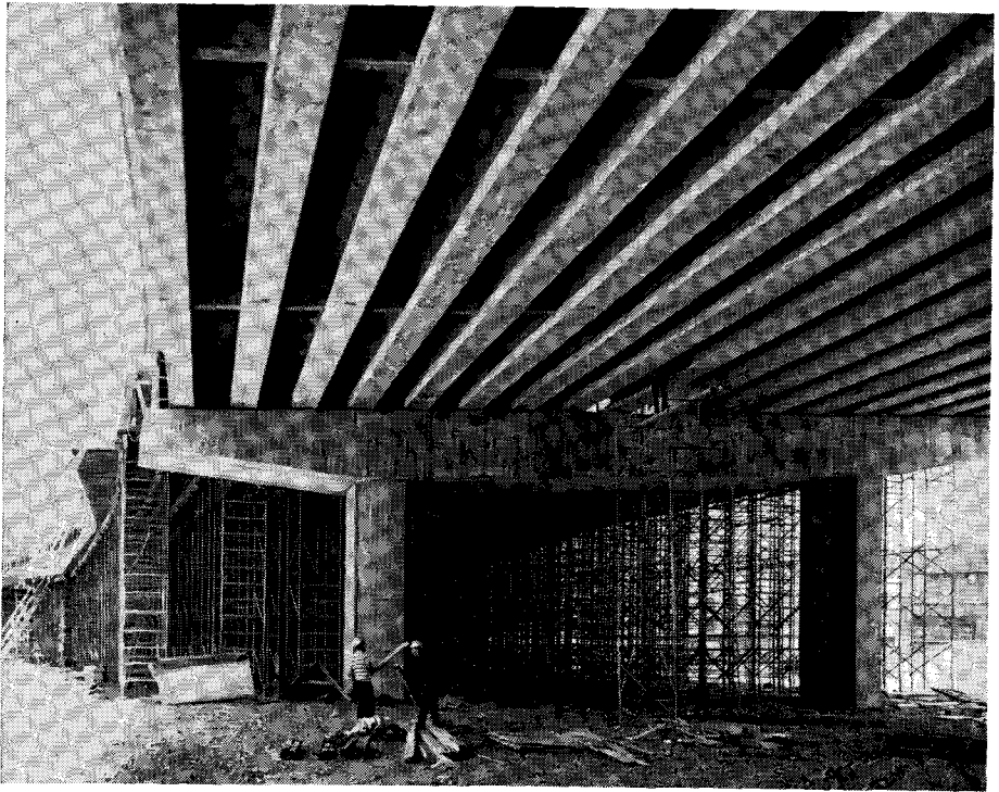
Fig. 10—A Portion of Bonaventure Autoroute Shows Cast-In-Place Box Girders in the Background with Prestressed Girders in the Foreground Span
