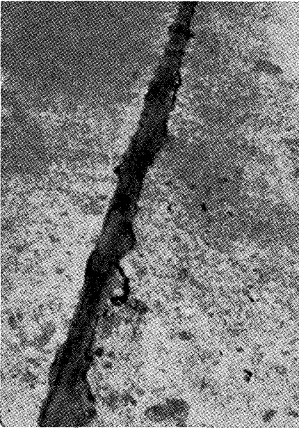
Fig. 4—Concrete Torn by High-Modulus Sealant.
