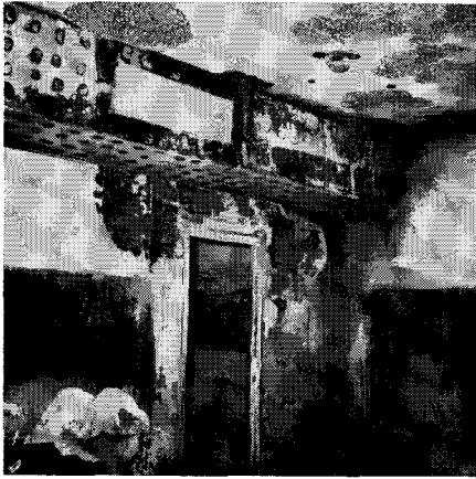
Fig. 7—Steel stud partition having metal lath and plaster between Rooms 20 and 21 was completely bare of plaster around top of steel door frame which was warped.
