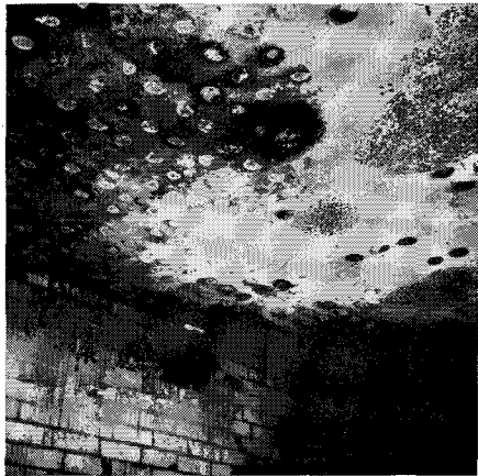
Fig. 10—Clay brick east wall was spalled to a depth of ¾ in. over 2-ft. diameter spot even though the adjacent lightweight concrete ceiling slab did not spall.
