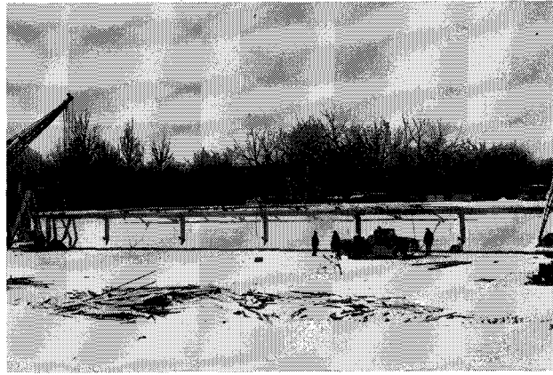
Fig. 5—Preparing a girder for movement with transporting frames and dozers at each end.
