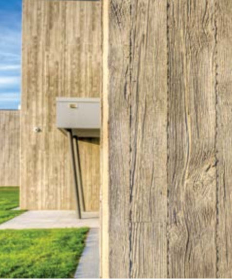
One of the building's most unique design elements is the application of the wood grain formliner. The insulated precast concrete wall panels are load-bearing with a barn board finish selected to give the concrete a modern appeal and feeling of warmth. Photos: Craig Van Wieren, Modern[edge] studios.
