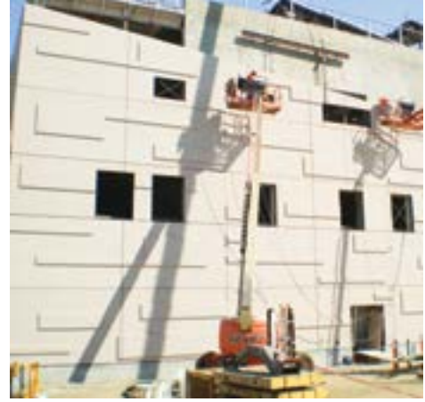
The panels were cast and delivered to the site for immediate erection as the schedule required, eliminating site congestion. Photo: Clark Pacific.
