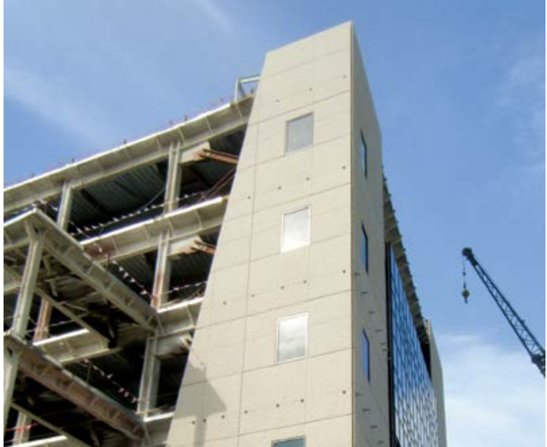
Some of the panels include a sloped right-hand face to fit against the slope of the curtain wall's left-hand side. Photo: Clark Pacific.
