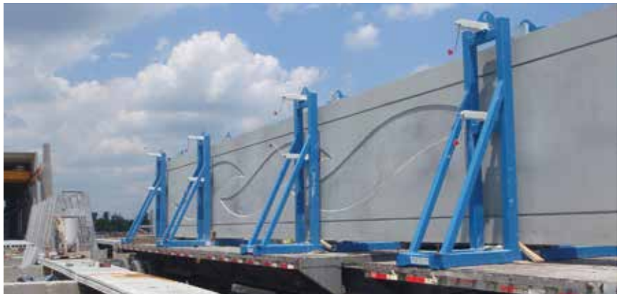
Spandrels with the port's logo cast into them are shown. Two crews were used to shorten the schedule and keep it off the critical path of construction for the terminal being built. Photo: Canaveral Port Authority.
