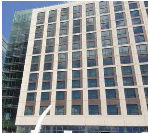
Figure 1a Hyatt Regency expansion, Tysons Corner, McClean, Va. All figures and photos: RTKL Associates.
