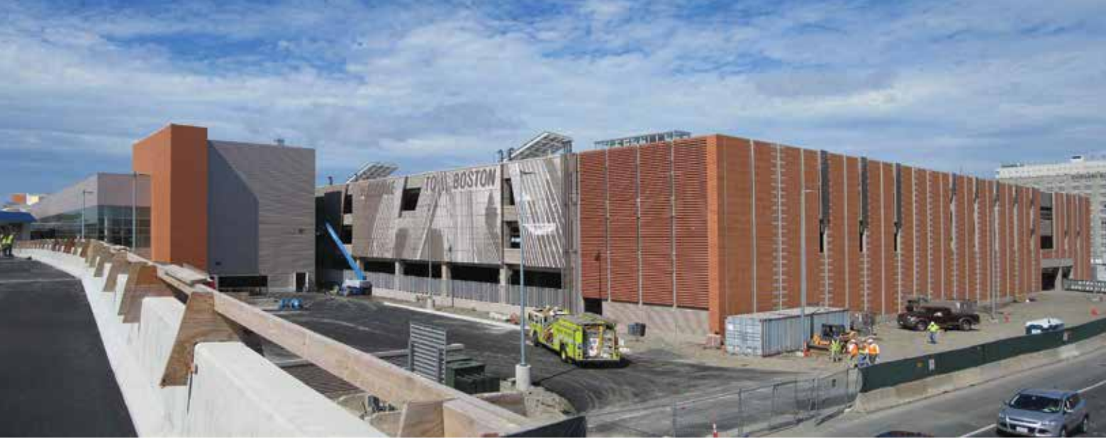
Precast concrete components created 60- by 60-foot bays for the CONRAC facility at Logan International Airport in Boston, Mass. Structural H-frames supported loads along the perimeter, with interior moment frames used between columns and tees. Terra cotta veneer was applied to the exterior, its first use in North America on structural components. Photo: Fennick McCredie Architecture.
