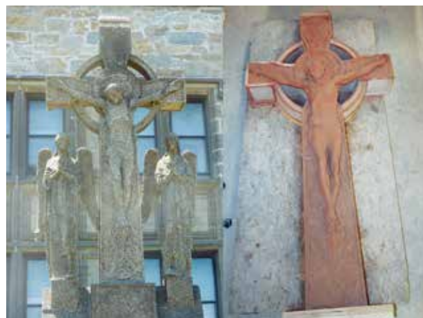
The original crucifix statue, shown in its heavily weathered state, had to be resculpted in clay (right) to create a mold so the piece could be recast in precast concrete.
