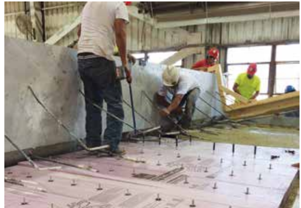
The panels’ thermal efficiency was a key advantage both in minimizing trade congestion and time as well as for meeting energy goals.
