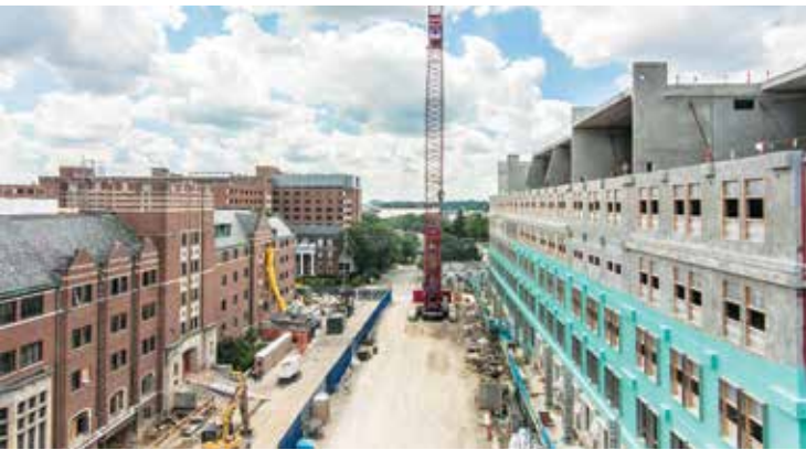
Because of the tight site with an adjacent project also underway, the precast concrete components were delivered on a just-in-time basis and erected through two shifts.
