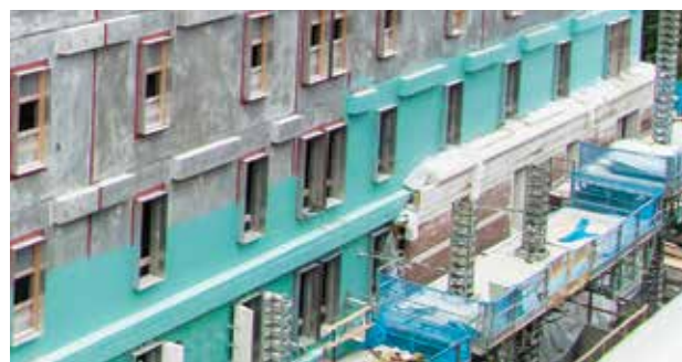
Fabricating the panels on a fast-track basis through the winter gave administrators time to select brick that matched nearby buildings that could be installed in the spring.
