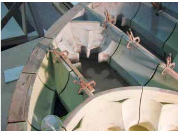
Each window tracery was recast as two back-to-back pieces rather than the 17 individual pieces in the originals. The traceries were installed and center mullions and surrounds were installed.
