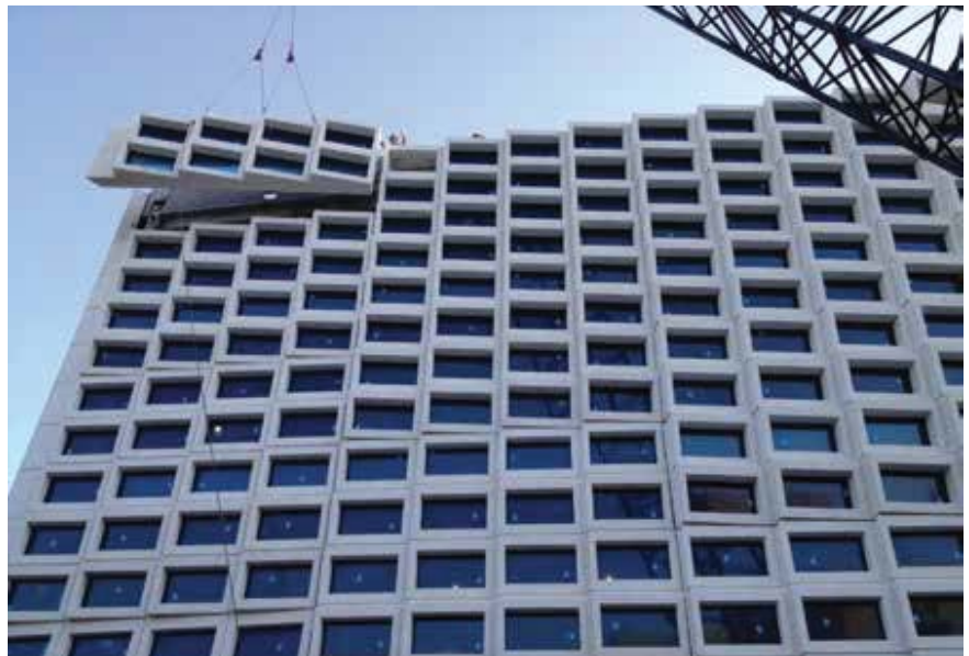
The glazing contractor installed the windows in the precast concrete panels and caulked them in the precaster's plant, which reduced safety concerns and boosted productivity. It also allowed the windows to be water-tested at the plant and again at the site.
