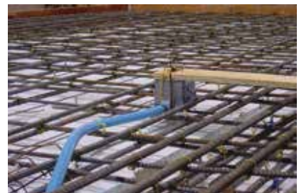
Installing electrical conduit and boxes involves pre-bending the metal or plastic conduit to the desired shape and installing it in the casting bed already connected to the electrical boxes. Photo: Gate Precast Co.
