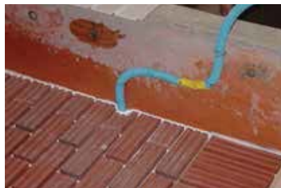
Electrical contractors coordinated their needs with workers at the Gate Precast Co. Ashland City, Tenn., plant to ensure the electrical installation moved smoothly. Photo: Gate Precast Co.
