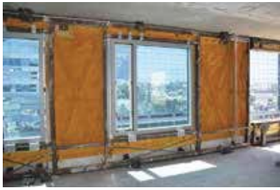
The panels feature 2 inches of NCFI spray-foam insulation on their back side. Special forms produced sheets of insulation that were cut into strips and used to form dams at breakout locations.
