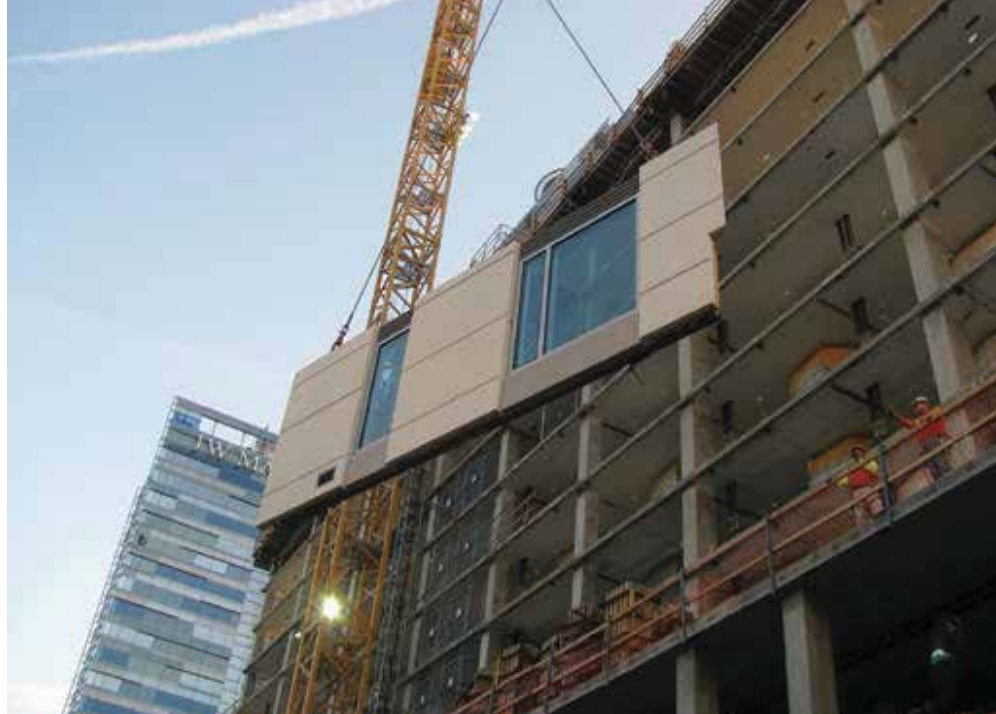
The composite panels erected on the LA Live Marriott hotel had light-gauge steel tubes and galvanized pins added so window crews could install windows at the precaster's plant prior to shipping the panels. In all, 484 pre-insulated, preglazed panels, encompassing 119,000 square feet, were erected. Photo: Clark Pacific.
