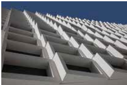
The panels feature integral sunshades in the form of protruding boxes around the window openings, which had angles varying from 0 to 15 degrees.
