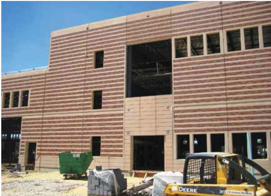
Selecting a brick to provide the desired aesthetic for the WMATA campus wasn't difficult, but the choice had to meet the district's Architectural Review Standards Board's requirements.
