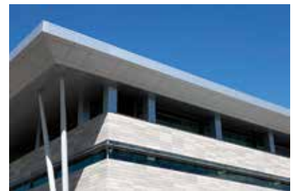
Terra-cotta tiles that were 1 3 / 16 inches thick were embedded into insulated precast concrete panels to clad the Public Safety Building in Salt Lake City, Utah. The high-performance precast concrete panels provided both energy efficiency and protection from ballistic penetration. Photos: Benjamin Lowry, GSBS Architects.
