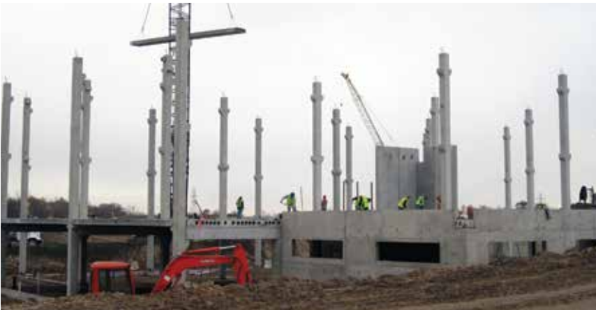
The precast concrete design proved to be 20% less expensive and saved months of construction time compared to a steel frame. Photo: Kerkstra Precast.
