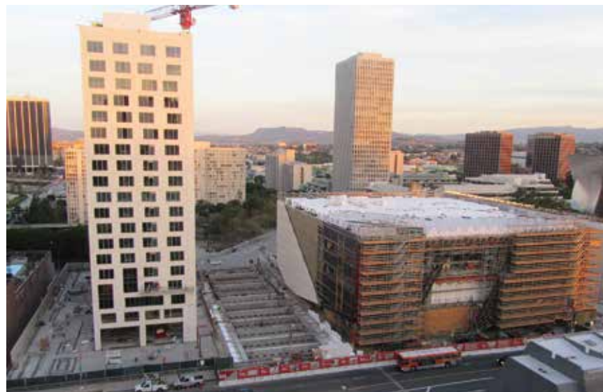
Field trips include site visits to buildings underway, including these three adjacent projects in downtown Los Angeles: the Grand Avenue Apartment tower, the Grand Avenue bridge park, and the Broad Museum.
