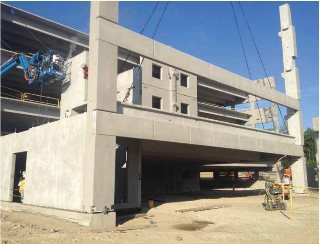
The first phases of the $500-million University Station project features 550,000 square feet of retail space and a 350-luxury residential development. The residences will wrap about a central precast concrete parking structure.
