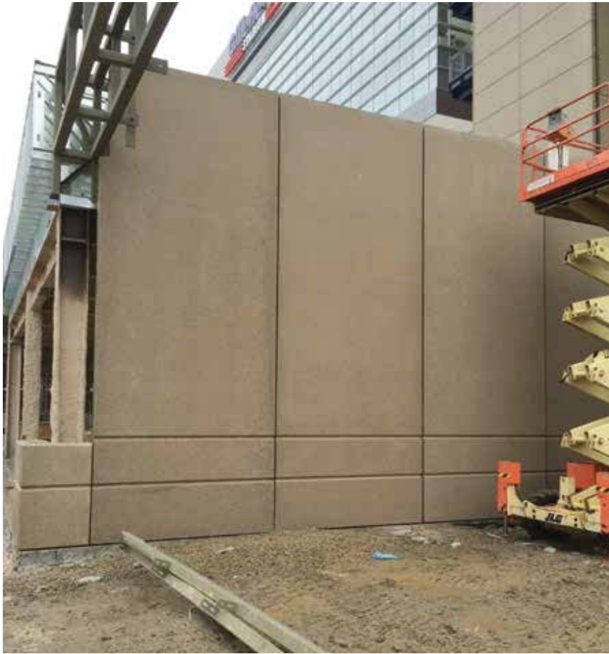
Eighty precast concrete components, including architectural panels and planter wall curbs, helped the two-story, 25,000-square-foot addition to Gillette Stadium match the existing structure and complete construction faster.
