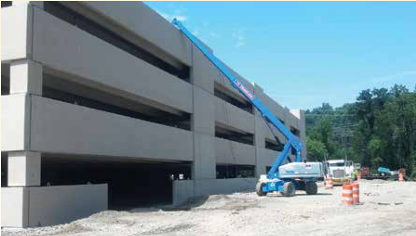
BioMed Realty Trust is currently constructing a 246,000-square-foot total-precast concrete parking structure to house 823 cars on its campus. To be completed in October, it will serve two new facilities being built and is clad with architectural precast concrete panels.
