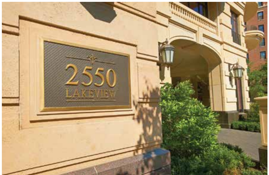
Black-granite and limestone veneer pieces were field-applied to the lower three levels of the building, providing visual interest at pedestrian level. Photo: High Concrete Group LLC.
